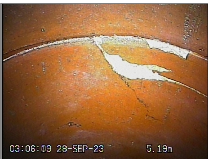
Fracture longitudinal at 1 o'clock
