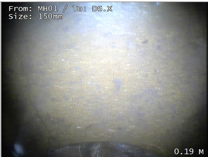
Line of drain/sewer deviates down
