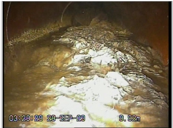
BUILD UP OF FOUL WASTE
