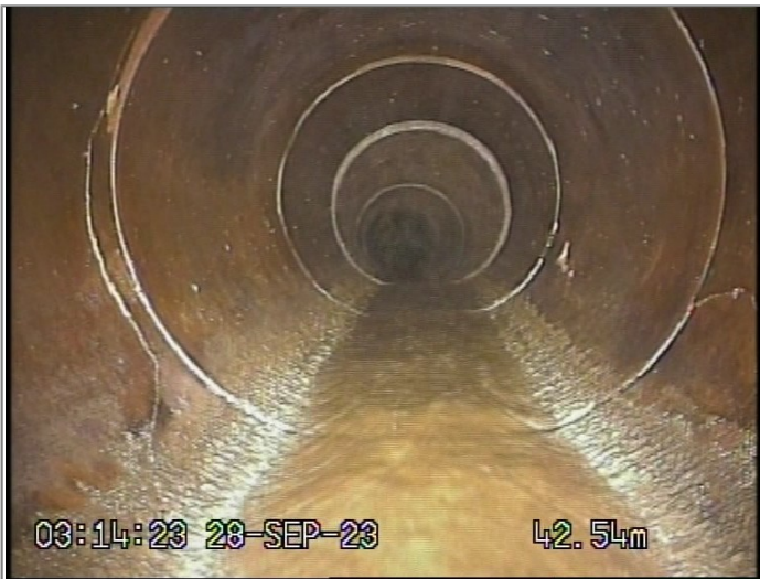
Fracture longitudinal at 4 o'clock
