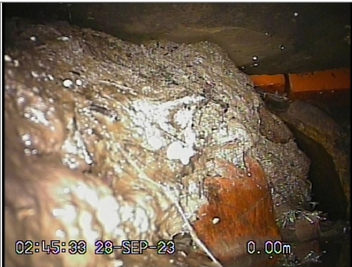
Settled deposits fine 75% cross-sectional area loss
