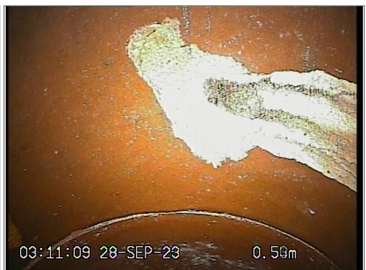
Hole in drain/sewer at 11 o'clock
