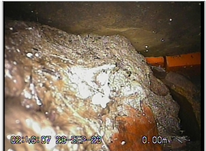
Survey abandoned - Remark: OBSTRUCTION - UNABLE TO PASS HIGH SILT DEPOSITS
