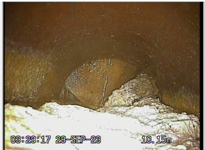
Survey abandoned - Remark: OBSTRUCTION - UNABLE TO PASS DUE TO HIGH AMOUNT OF SETTLED DEPOSITS IN PIPE - MH IN VIEW
