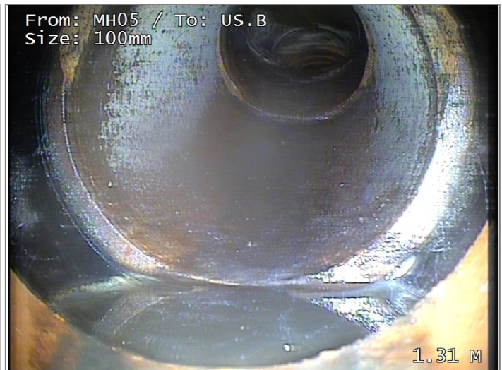
Line of drain/sewer deviates up
