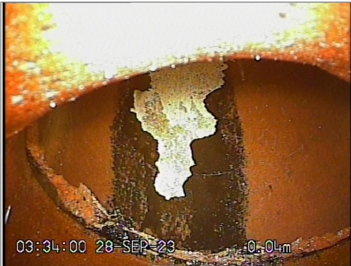
Line of drain/sewer deviates up
