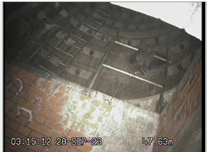
Finish node type, manhole, reference UU 1205
