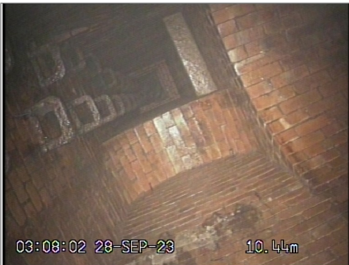
Finish node type, manhole, reference UU 1204
