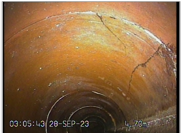
Fracture longitudinal at 2 o'clock
