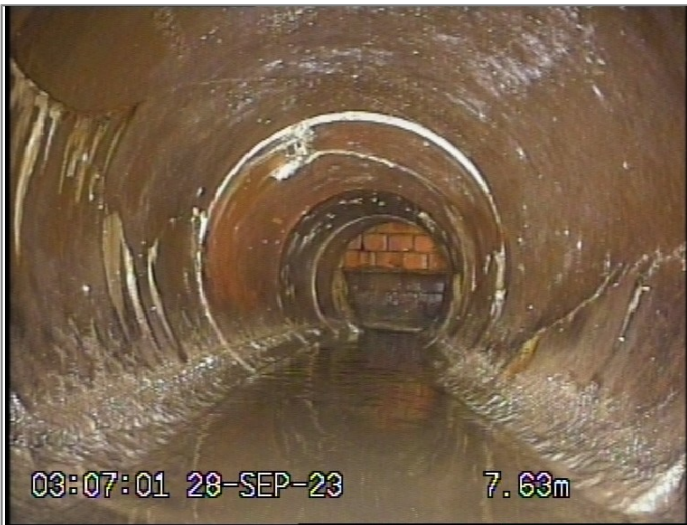
Fracture multiple from 3 to 3 o'clock, Start
