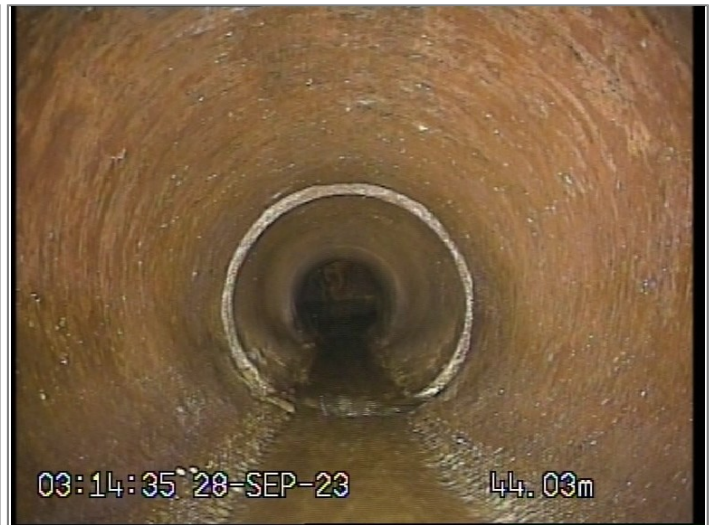
Line of drain/sewer deviates down
