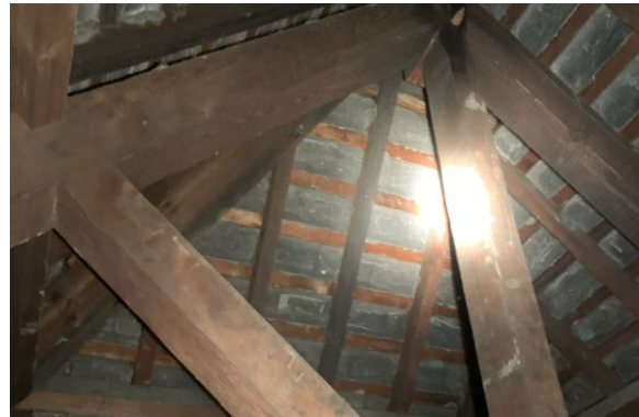
Picture 14 – Well sealed internals of R1
