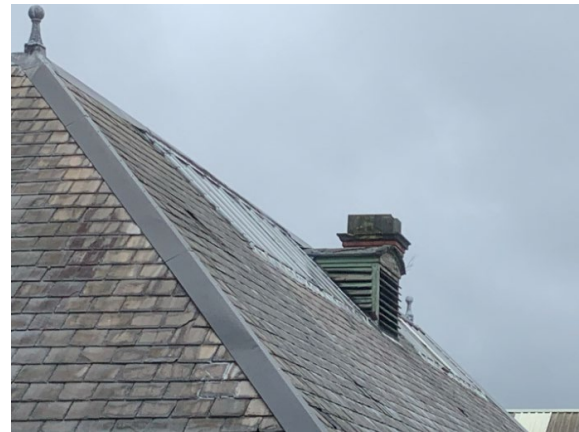
Picture 10 – Dilapidated dormer
