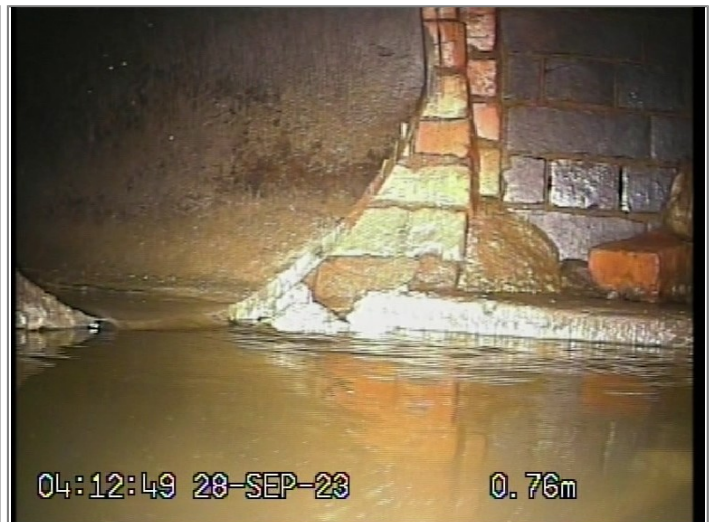
Line of drain/sewer deviates left
