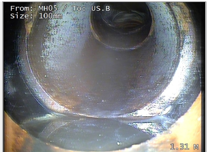
Line of drain/sewer deviates up
