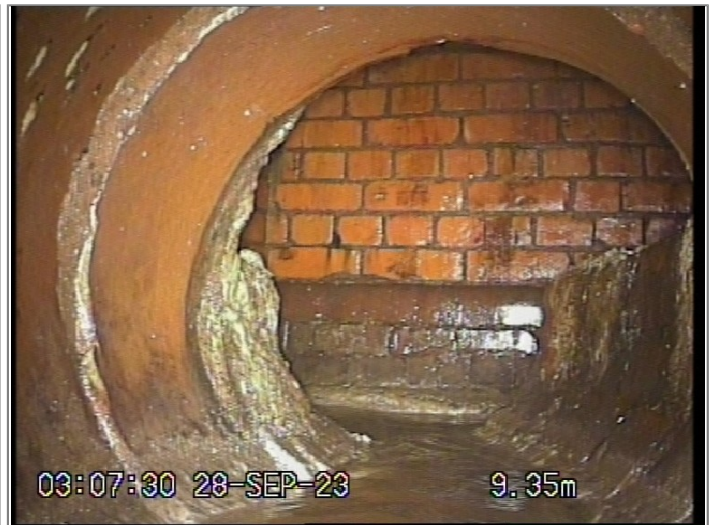
Fracture multiple from 3 to 3 o'clock, Finished
