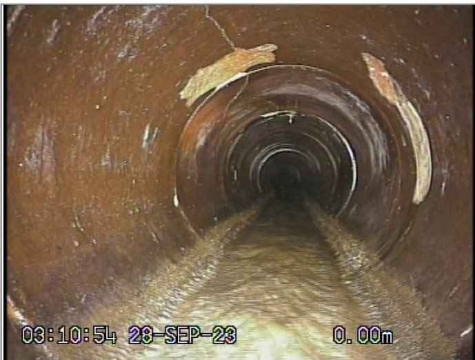
Fracture longitudinal at 12 o'clock, Start
