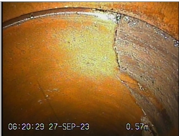
Fracture longitudinal at 3 o'clock
