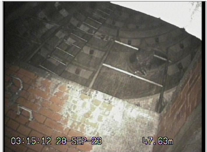
Finish node type, manhole, reference UU 1205
