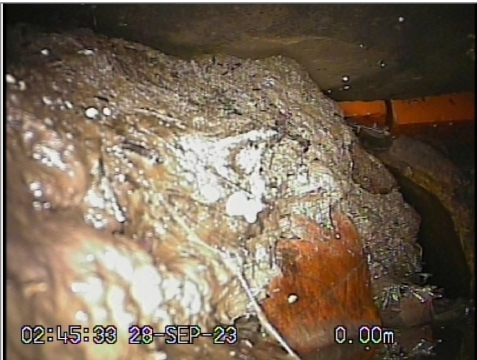
Settled deposits fine 75% cross-sectional area loss
