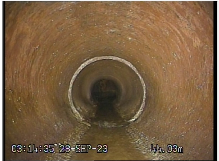
Line of drain/sewer deviates down
