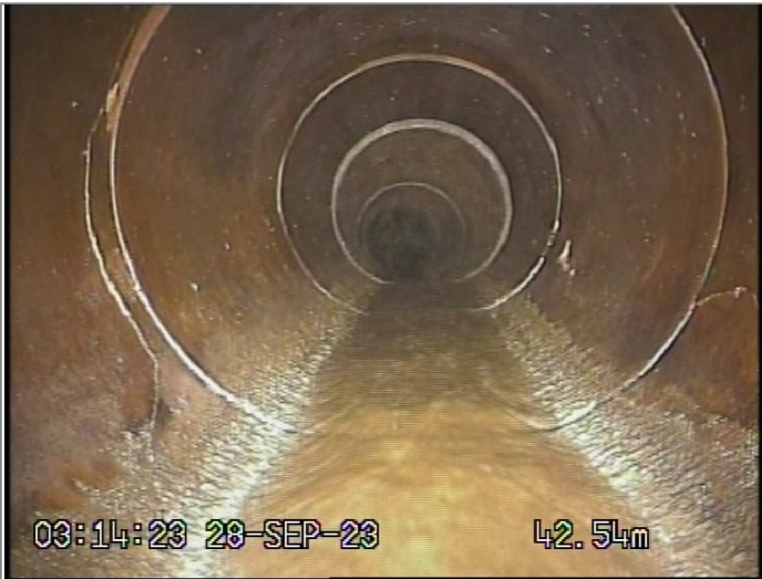
Fracture longitudinal at 4 o'clock
