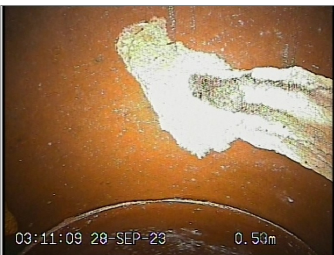
Fracture radiates from 2 o'clock
