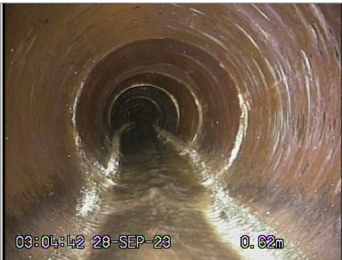
Line of drain/sewer deviates left
