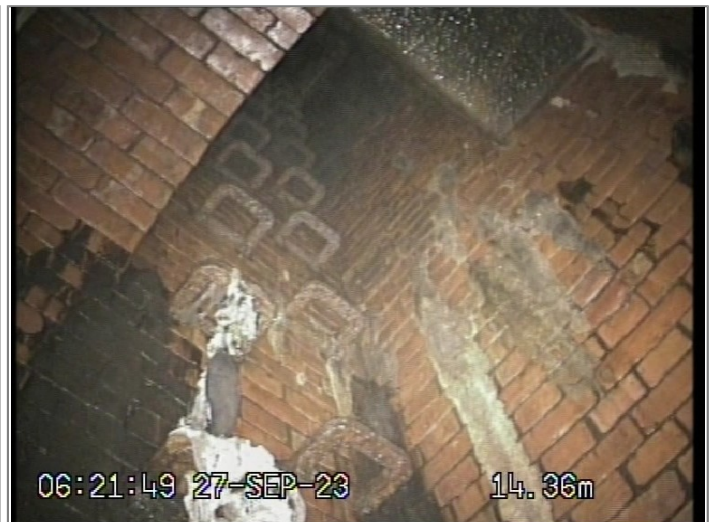
Finish node type, manhole, reference UU 1203
