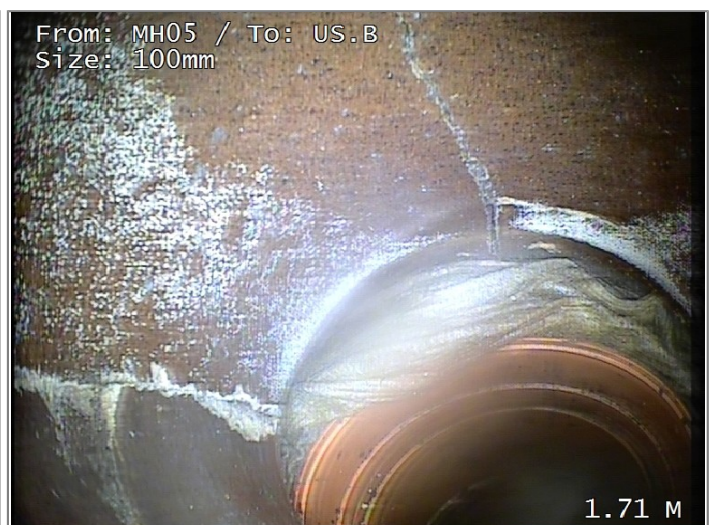
Fracture longitudinal at 8 o'clock
