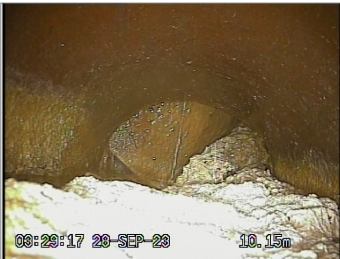
Other settled deposits 25% cross-sectional area loss - Remark: FOUL WASTE, Finished
