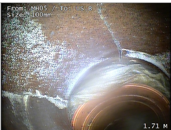
Fracture longitudinal at 12 o'clock
