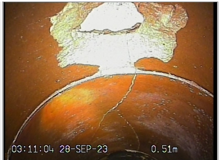
Fracture radiates from 11 o'clock
