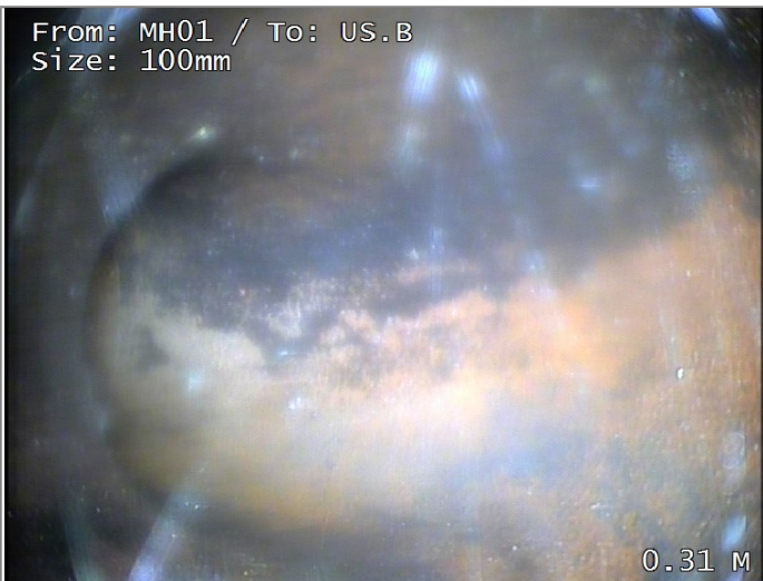
Line of drain/sewer deviates left
