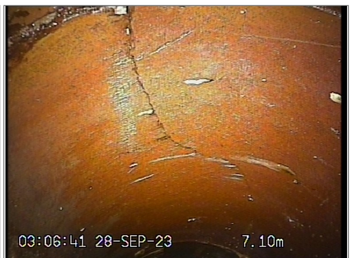
Fracture longitudinal at 10 o'clock
