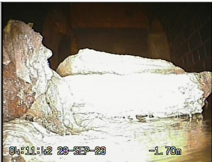
Settled deposits coarse 25% cross-sectional area loss
