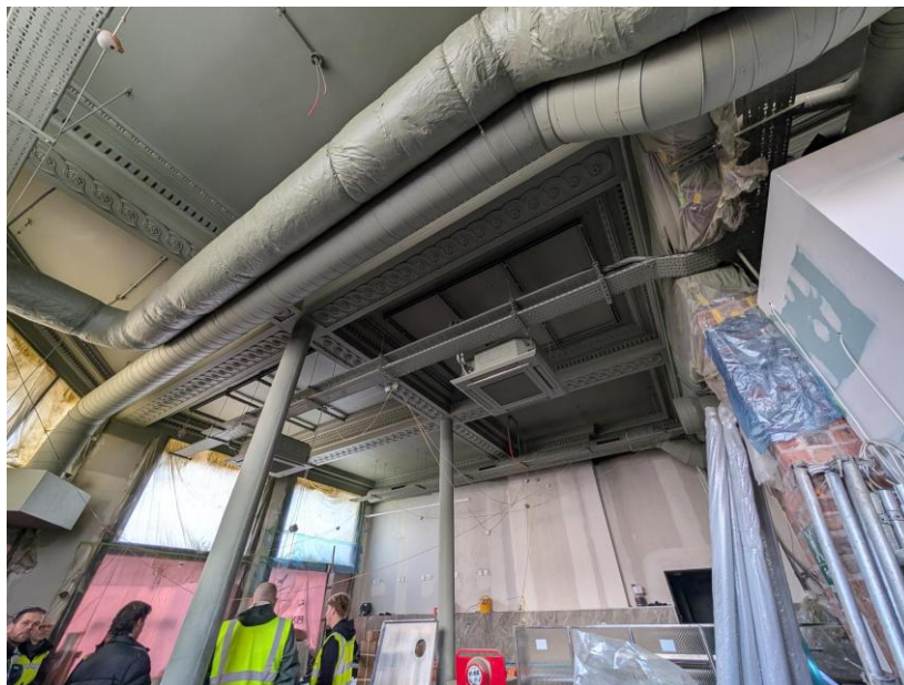
(Unauthorised M&E, plant, servicing and associated equipment indicates level of harm)
