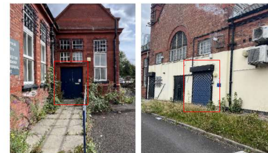
D.EXT.01 Front door to be replaced with new doorset to meet current thermal and security requirements
