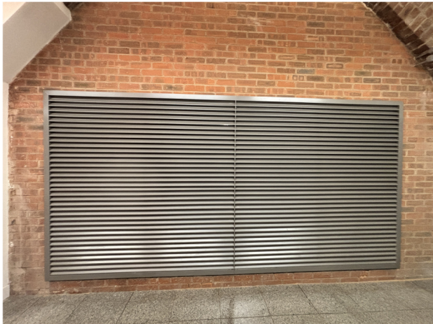
PREVIOUS NON-HISTORIC BRICKWORK INFILL WALLS TO ARCHES
