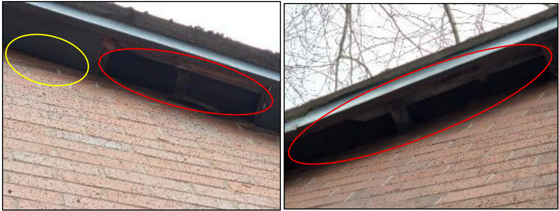
Photograph 5 (left) & 6 (right) showing gaps in soffit boards in northern elevation
