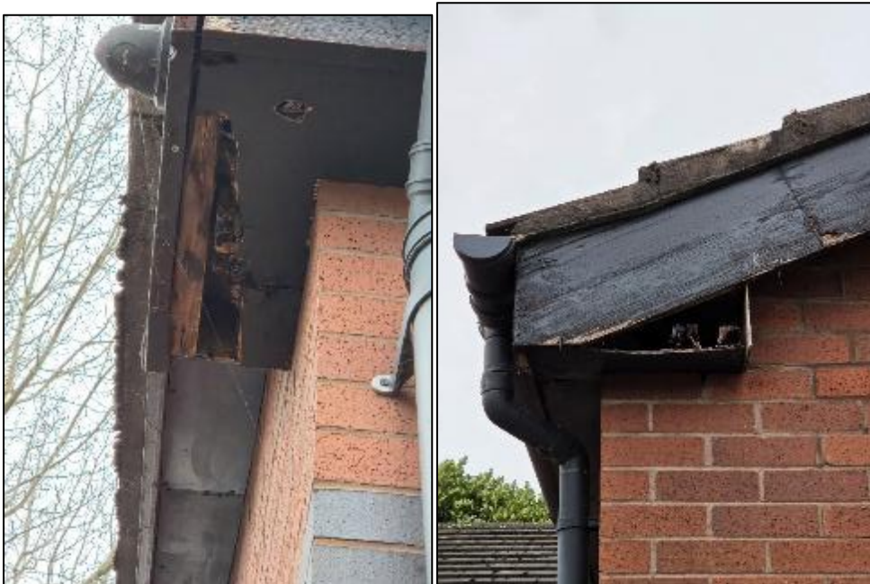
Photograph 7 (left) & 8 (right) showing gaps in soffit boards in southwestern and southeastern corners
