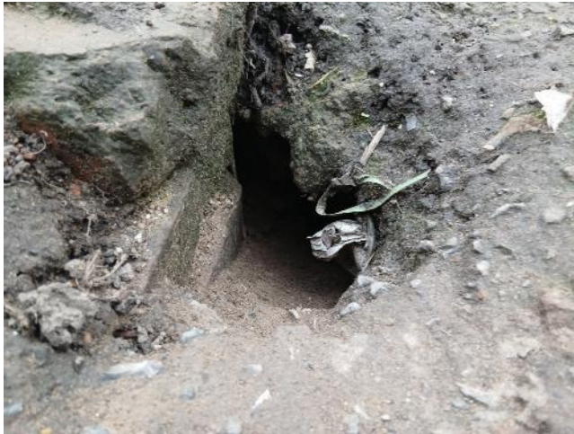
Photo 5: Small hole ~10cmx10cm at eastern section of the site
