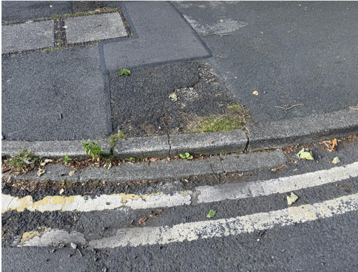
Crack in kerb and tarmac patch repair.
