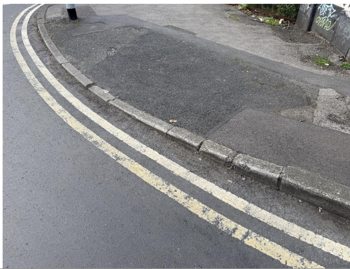
Damage to kerbs.
