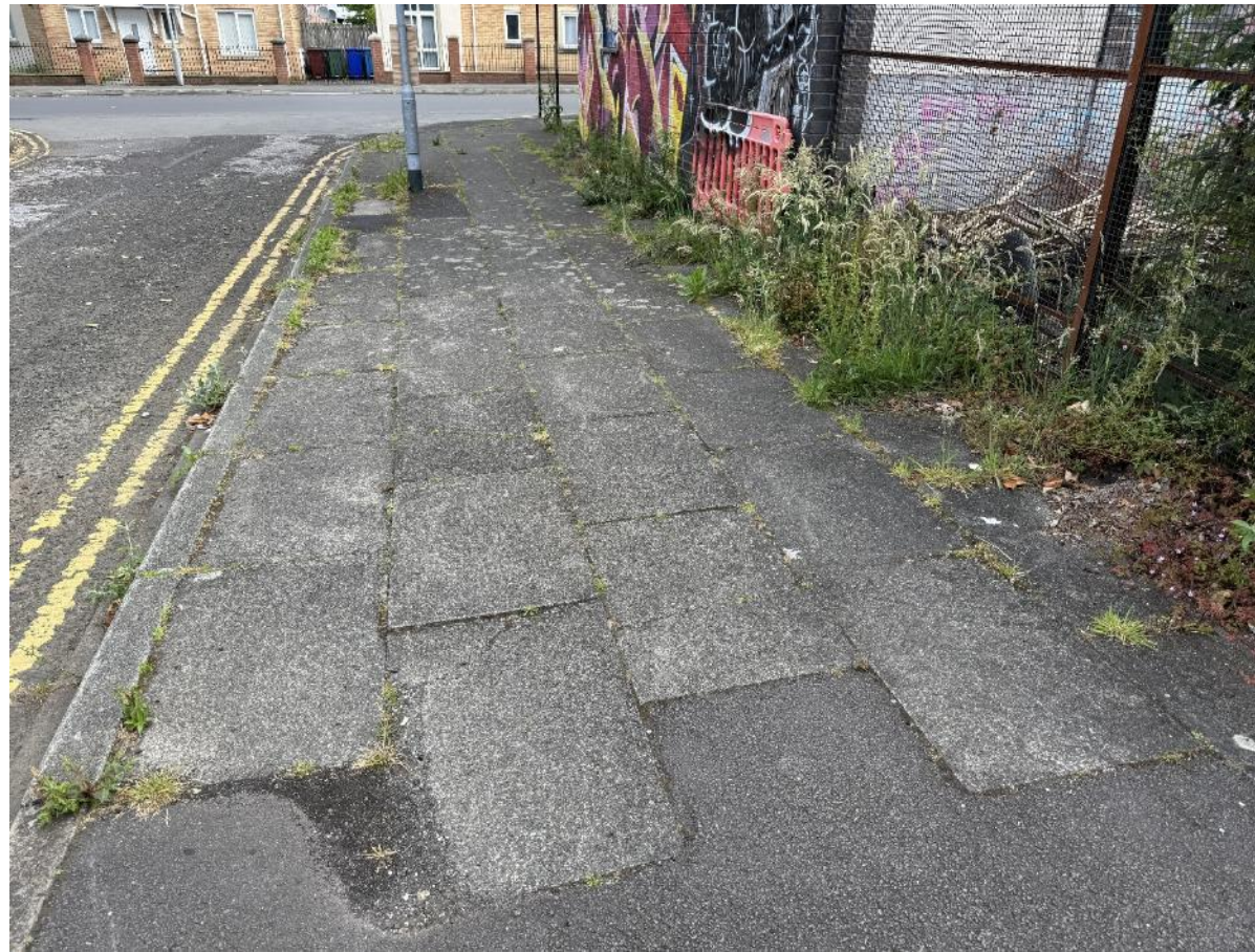
Broken and sunken flags.
