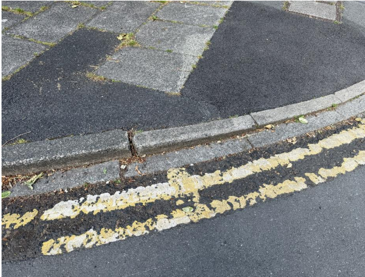
Kerb damaged and sunken.
