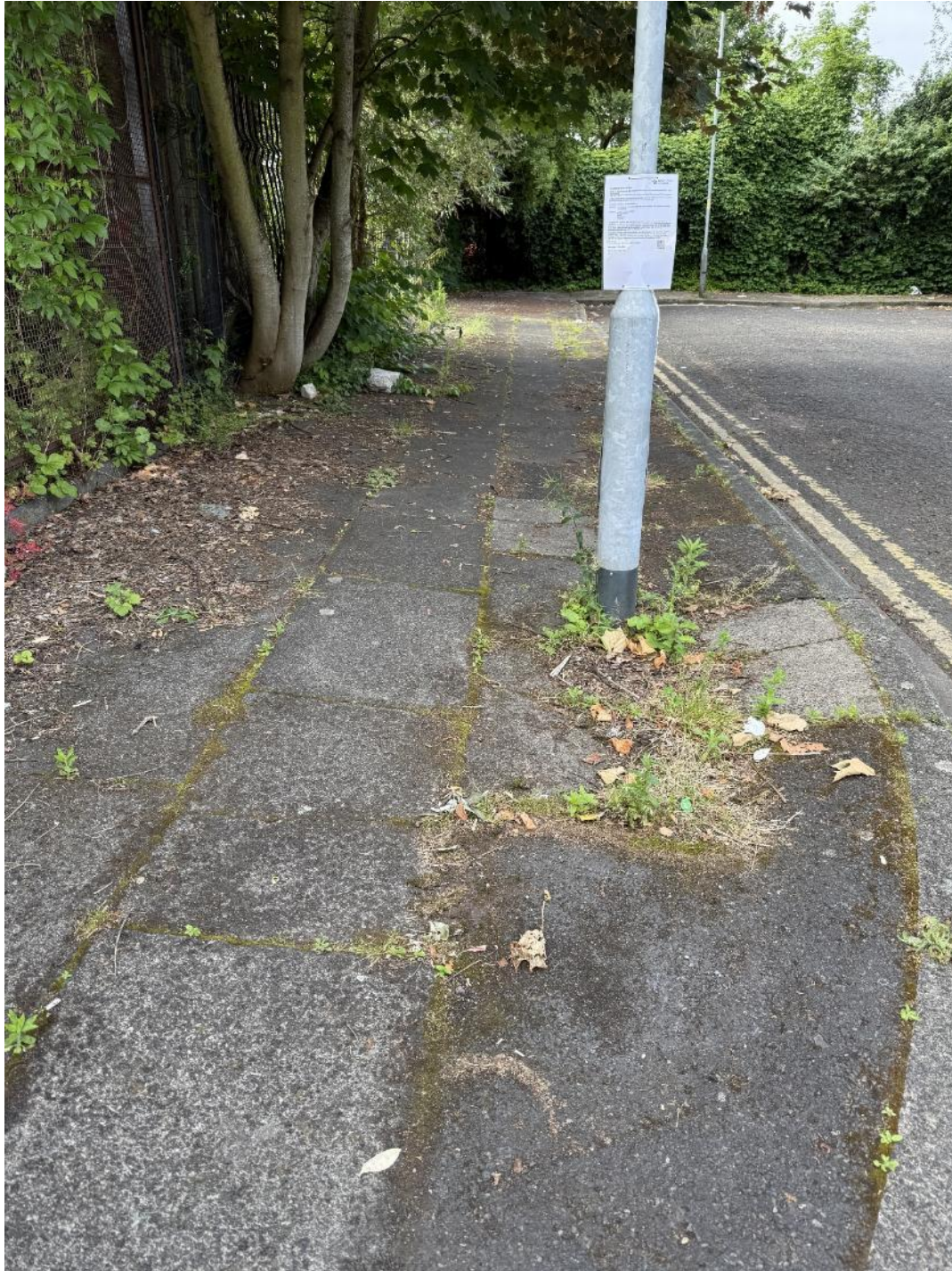
Concrete slabs broken and severely sunken.
