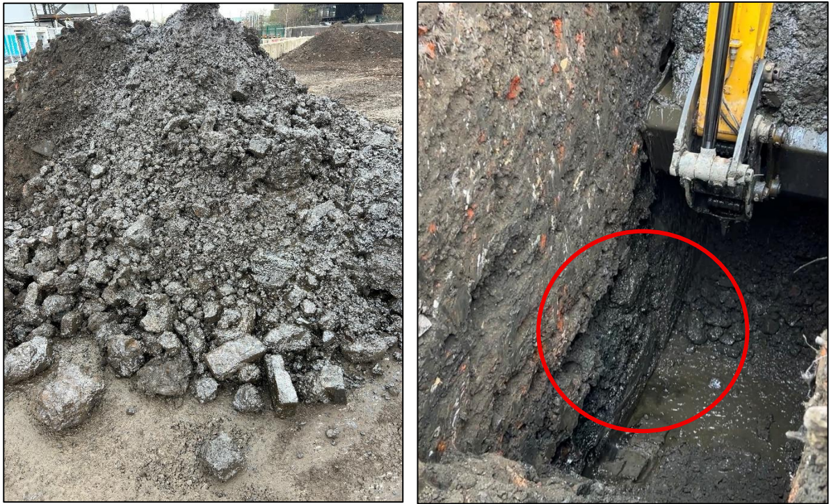
Figure 7: Photographs of Made Ground where strong hydrocarbon odours and sheens were recorded (TP303, left and TP309, right)
