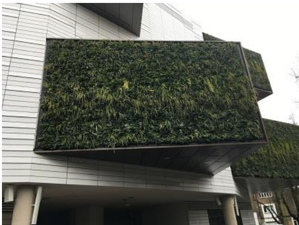
Figure 6—7 Modular green walls (Lord's Cricket Ground, London)
