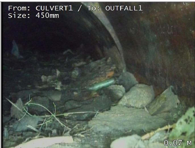
Settled deposits coarse 60% cross-sectional area loss, Start
