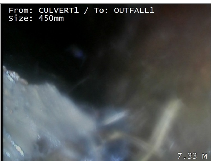
Survey abandoned - Remark: 75% FULL DEBRIS AND ROOTS
