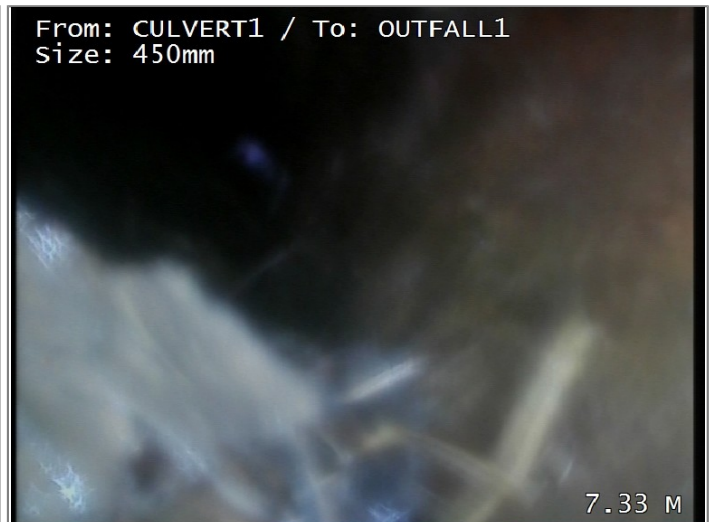
Settled deposits coarse 60% cross-sectional area loss, Finished
