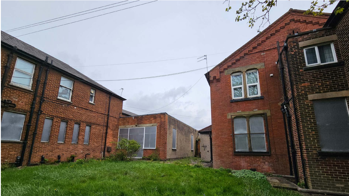
View 03 - Partial south elevation of St Anne's House (with lower quality extension to the right) and single storey blocks with damp issues haphazardly connecting into 1960s Courtyard Building (to the left).
