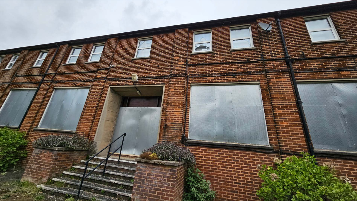
View 05 - Southern Elevation of 1960s Courtyard Building - Showing vandalised windows which have caused additional damp and rot issues internally of the building.
