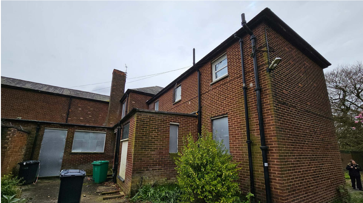
View 06 - Partial north elevation of 1960s Courtyard Building - Showing complex arrangement of building forms that lead to a convoluted layout of small cellular rooms within.
