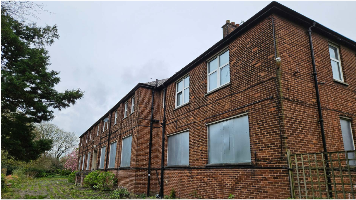
View 04 - Southern Elevation of 1960s Courtyard Building - Showing the expanse of uninsulated external walls and weathering of the delapidated unoccupied building.
