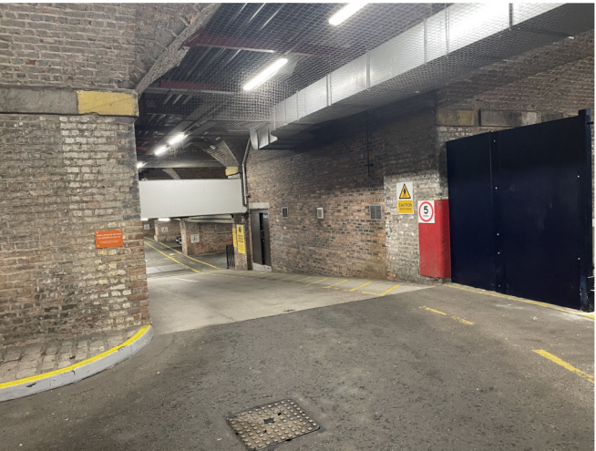
PREVIOUS NON-HISTORIC BRICKWORK INFILL WALLS TO ARCHES
