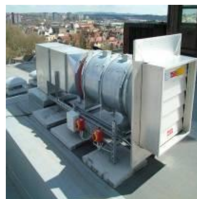
Typical "Colt Shaft" fan set
