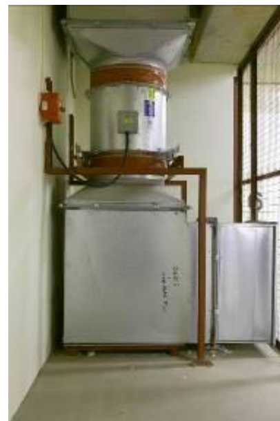
Typical car park extract fan system
