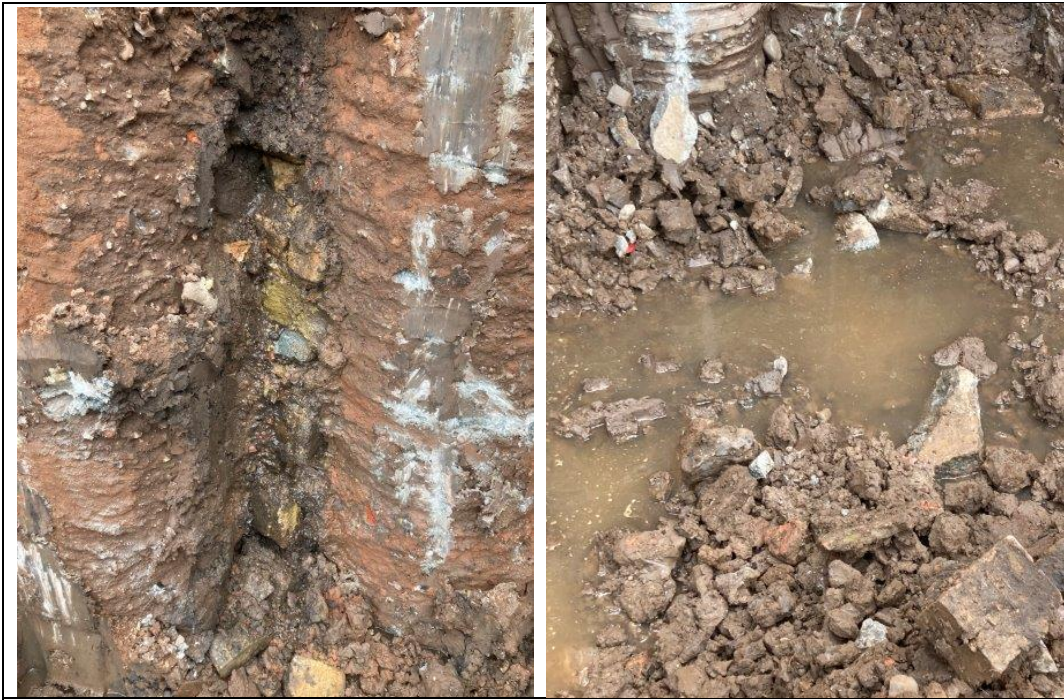
Water leak through augured piles
