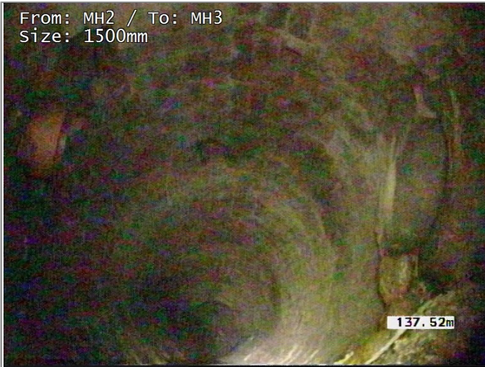
Connection other than junction at 3 o'clock, diameter 300mm
