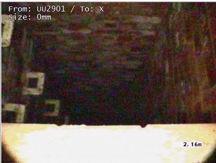
Survey abandoned - Remark: SEWER DEPTH ARROUND 12 TO 15M DEPTH
