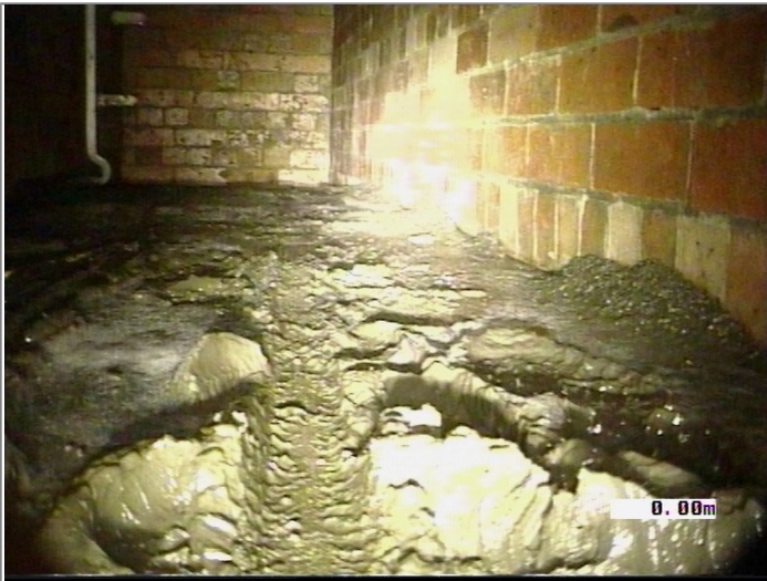
Start node type, manhole, reference UU2901
