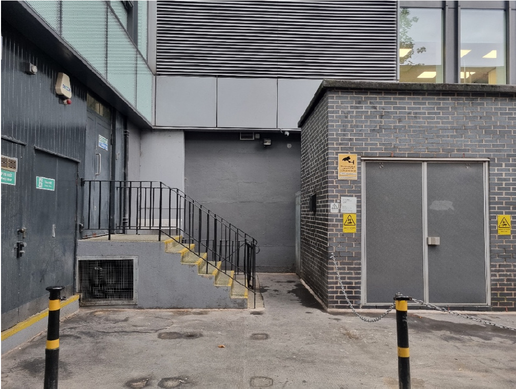
LEFT HAND SIDE OF EXISTING SUBSTATION ON BOOTLE STREET
