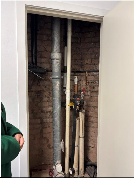
Figure 23: Existing M&E cupboard. Source: site visit, October 2025.
