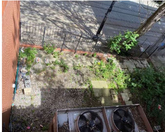
Existing plant compound , showing Co-Op retail unit chiller
