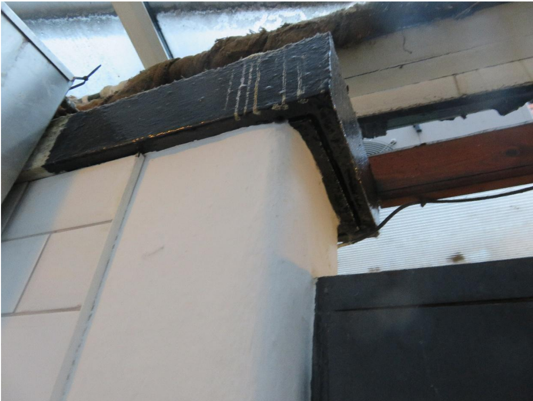
Urinal wall coping to be reused to over rear yard door, area above it has been covered over where once it was open with pvc glazing bars and polycarbonate sheet.
