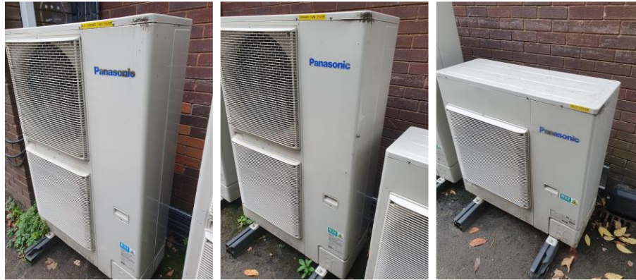
Figure 4 Condenser units' location
