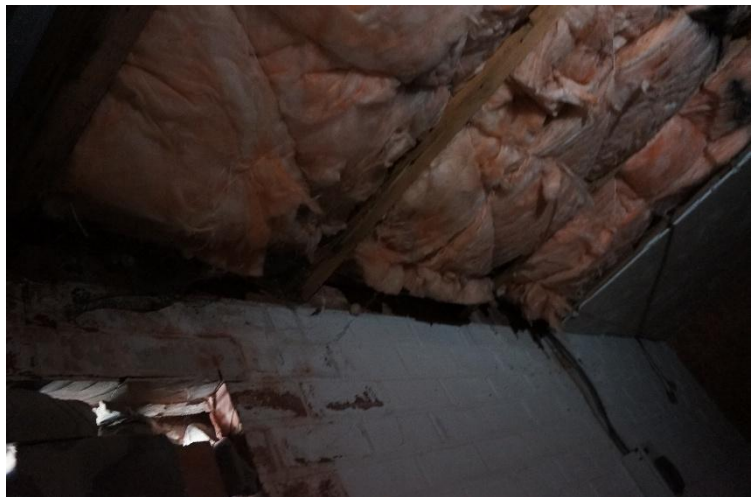
Figure 13: Example of exposed insulation, and gap to the outside.
