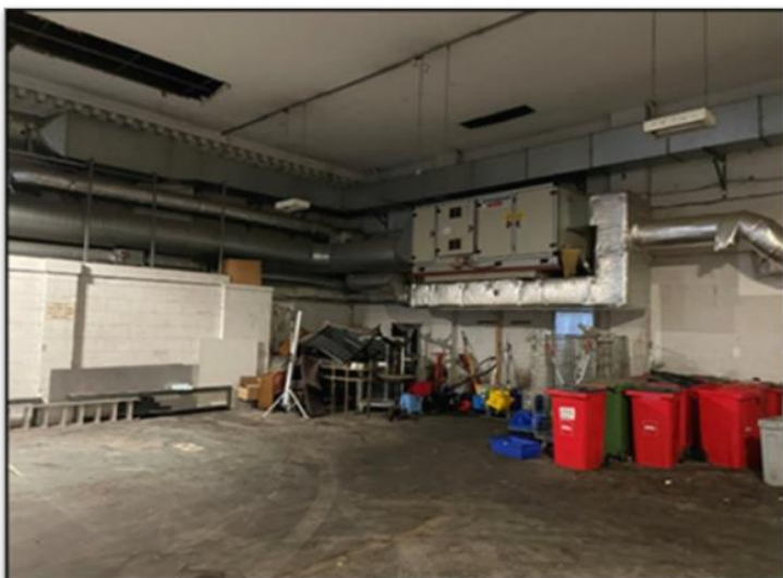
Photo 10. Interior of the carpark/service area with modern plant and suspended ceiling
