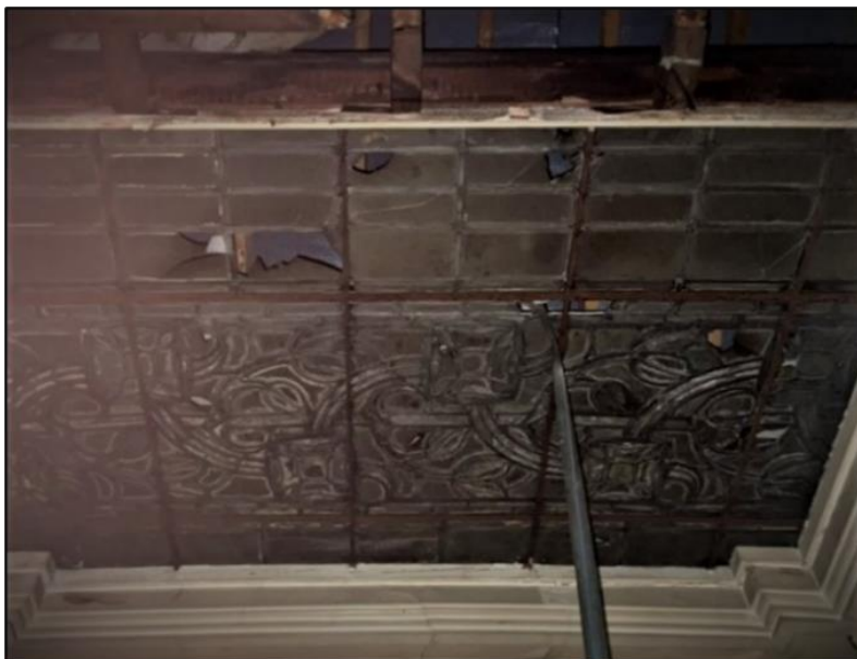
Photo 15. Remaining fragments of decorative glass from the Clerks' Room ceiling. Most of the ceiling was destroyed in the 1980's when the service yard was created, and a new slated pyramid roof built over.
