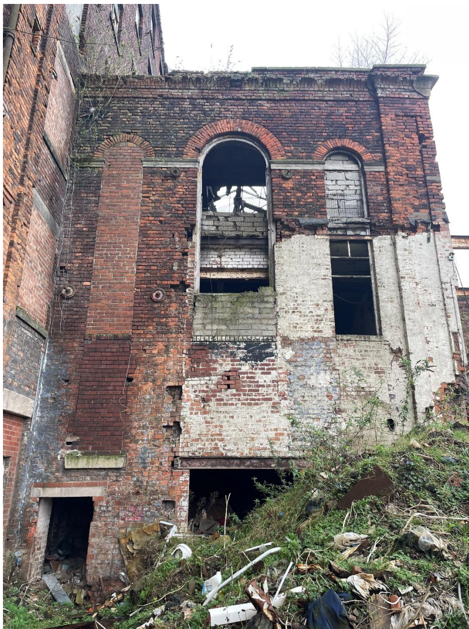
The north elevation of the engine house, illustrating the lower levels of the exterior masonry that requires paint removal to the north-west corner.
