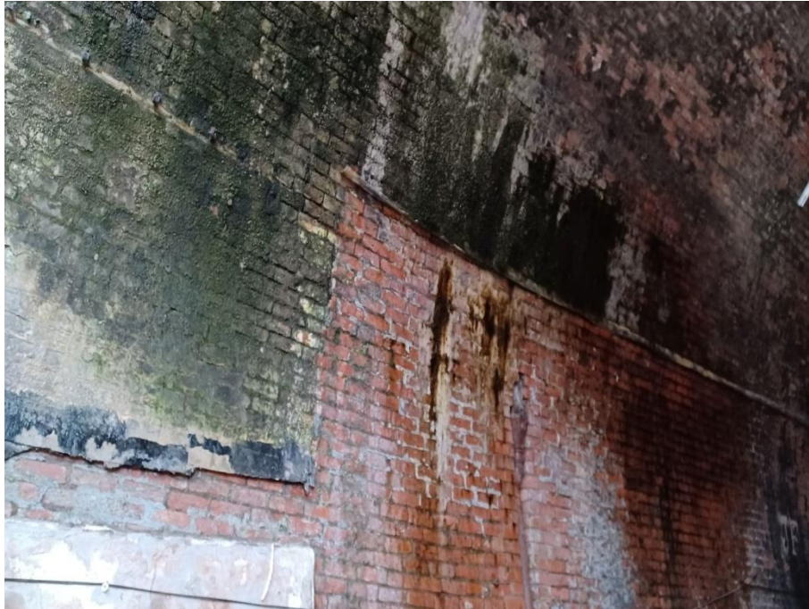
Photo 11: Moss growth, isolated open joints, and water staining / active ingress (dripping) to east face of span 1 arch barrel.
