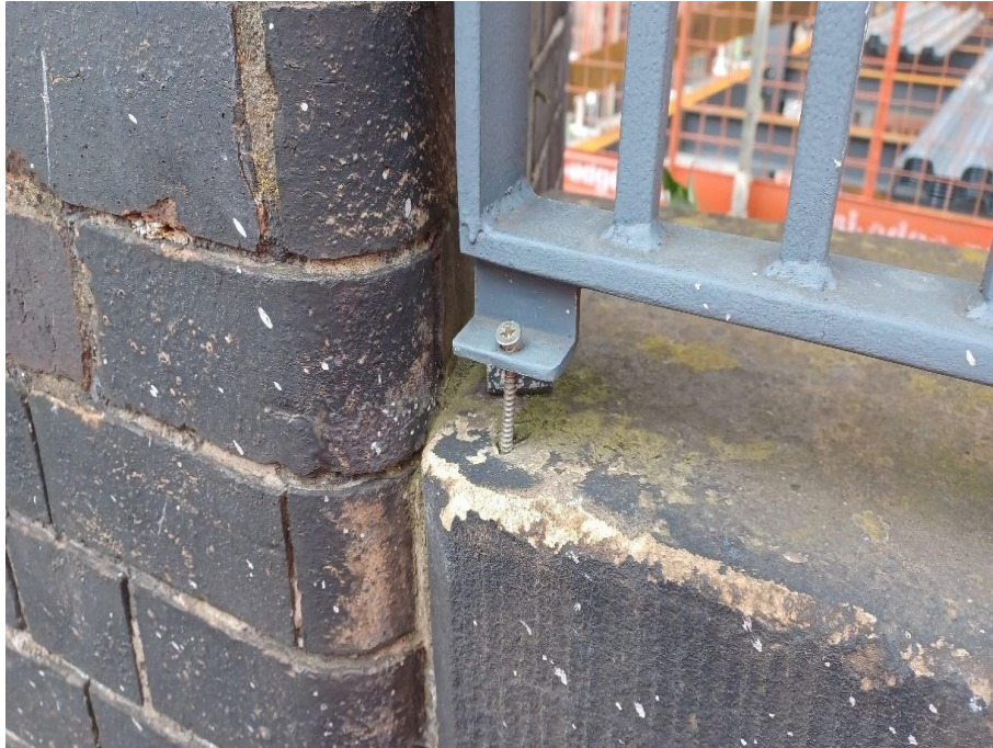
Photo 69: Loose fixing and railing at north end of north metallic parapet.
