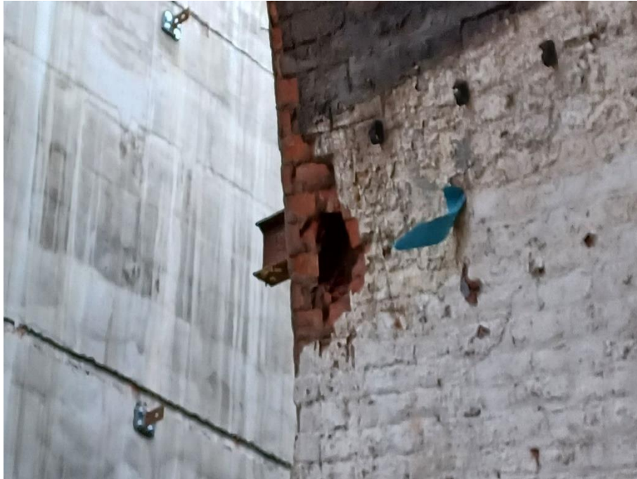
Photo 9: Spall to brickwork 1000x350x200mm to northeast quarter point of span 1 arch barrel.
