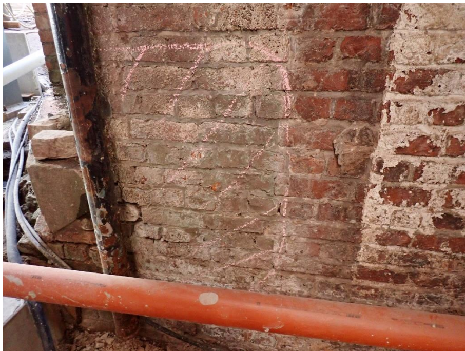
Photo 44: Area of hollow sounding brickwork 1000x500mm to north end of east abutment.
