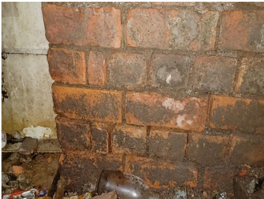
Photo 52: Area of open joints 500x300x10mm to south end of central pier.
