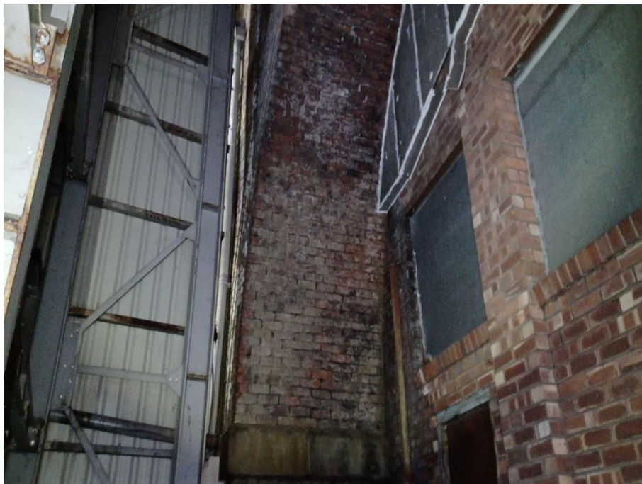
Photo 20: Water/leachate staining to southwest end of span 1 arch barrel.
