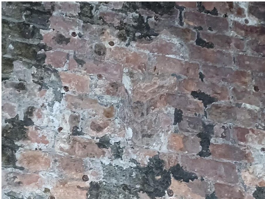
Photo 12: Spall 320x250x30mm to southeast end of span 1 arch barrel.
