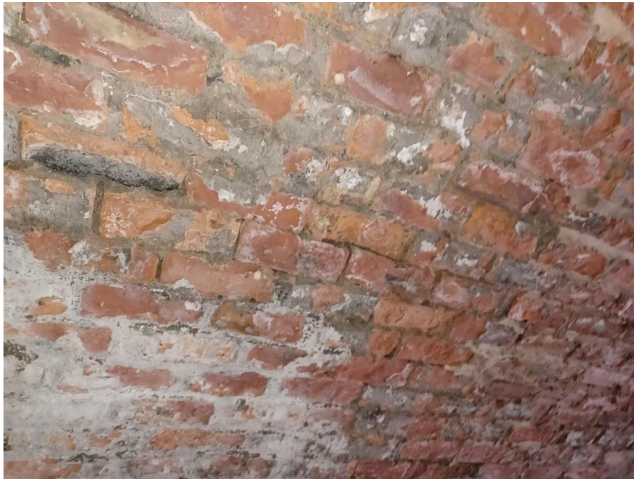
Photo 13: Area of spalling 1200x700x30mm and open joints at mid-span crown of span 1 arch barrel.
