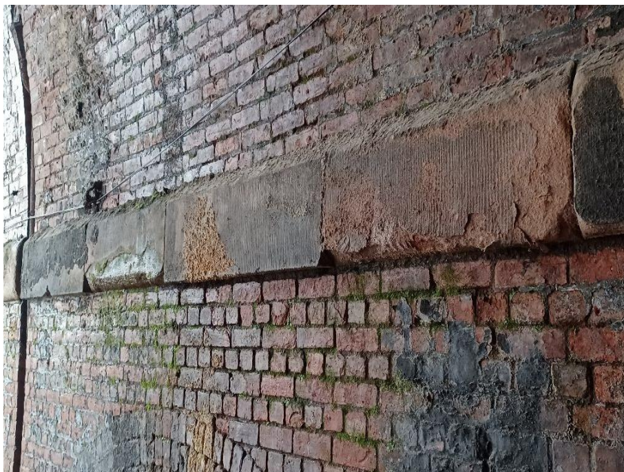
Photo 30: Isolated areas of surface spalling to mid-span of cill at west face of central pier.
