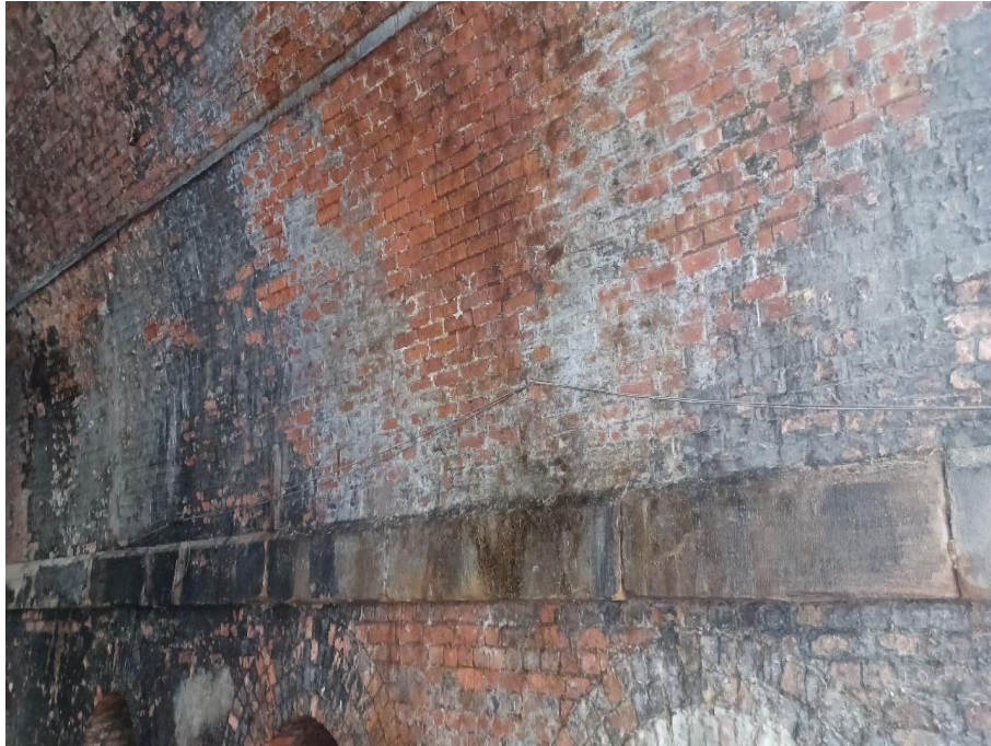
Photo 17: Area of wet friable mortar and active water ingress (dripping) 5000x7500mm to mid-span of west face of span 1 arch barrel.
