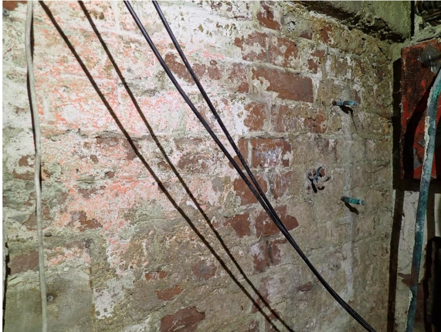
Photo 49: Staining and paintwork breakdown to north end of central pier east face.
