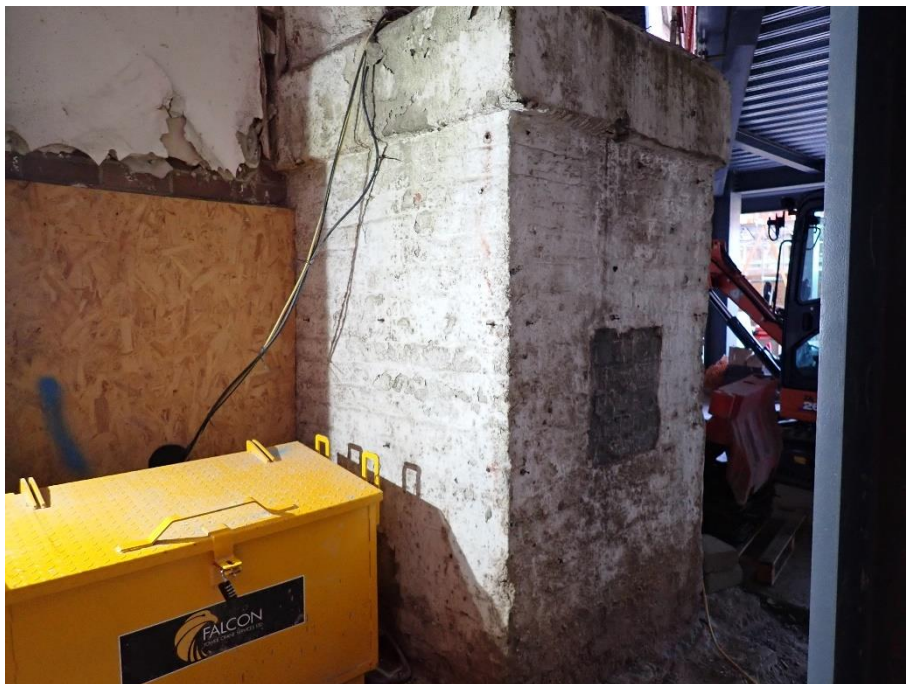
Photo 50: Paintwork breakdown and staining to north end of central pier.
