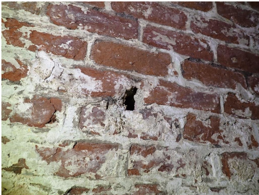
Photo 40: Hole (possible historic core hole) to east face south end of internal section of arch barrel span 2.
