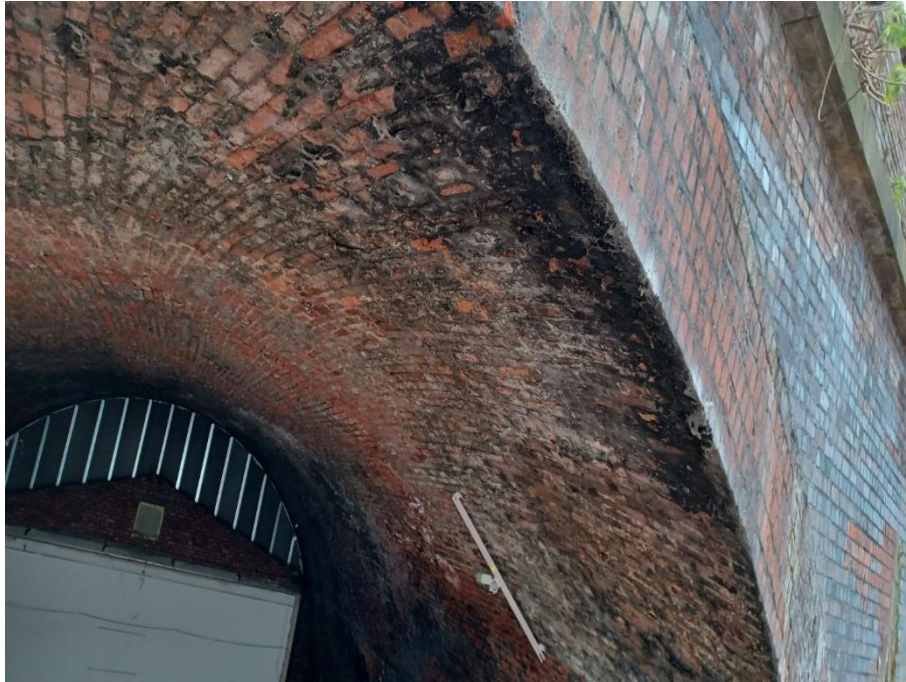
Photo 19: Area of hollow sounding brickwork 300mm wide from east to west springing's at north end of span 1 arch barrel.
