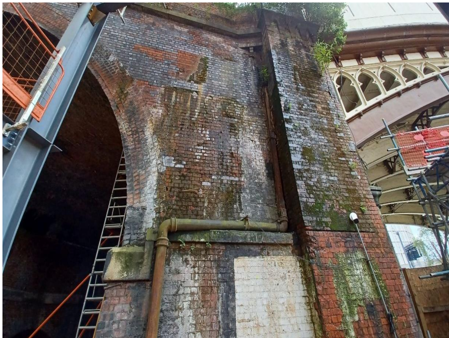
Photo 54: Water ingress (wet), isolated areas of surface spalling, and vegetation growth to west abutment and spandrel north elevation of span 1.
