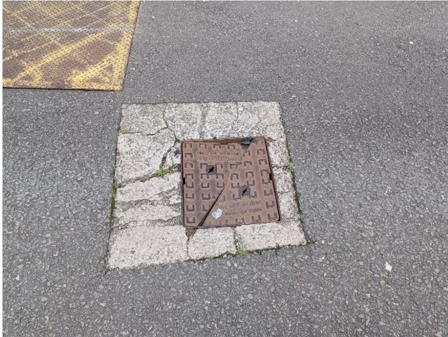
Photo 65: Sunken/displaced access cover in north carriageway.
