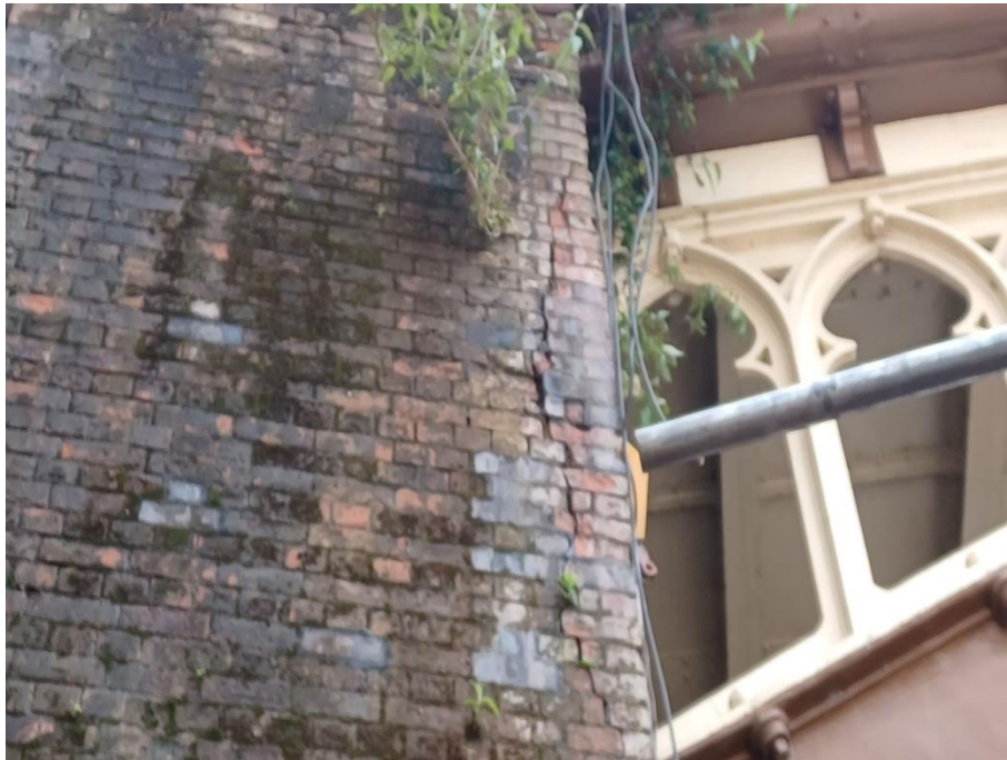
Photo 55: Vertical fracture up to 20mm with hollow sounding brickwork 2800x550mm surrounding fracture to west edge of west abutment north end.
