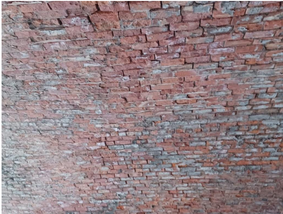
Photo 15: Area of surface spalling and open joints 4500x2500x25mm from east quarter point to west quarter point at north end of span 1 arch barrel.
