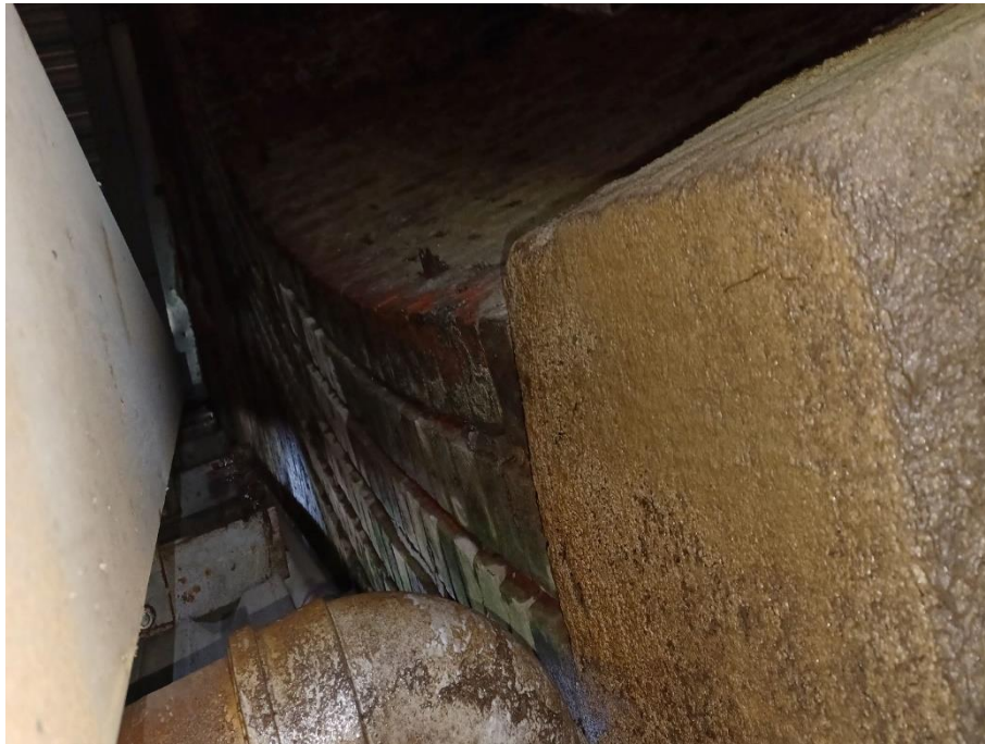
Photo 21: Area of open joints to southwest of face ring from springing up 2.2m by width of face ring and up to 20mm deep of span 1.
