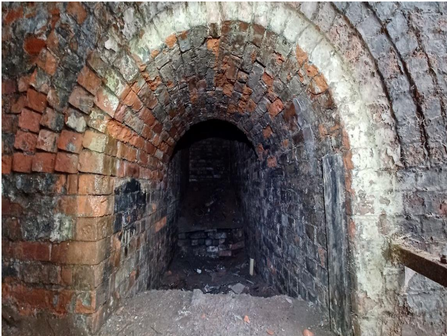
Photo 28: Open joints up to 30mm deep, wet friable mortar, surface spalling, leachate staining, and sodden brickwork to arch barrel of 5 th relieving arch from south end of west abutment span 1.
