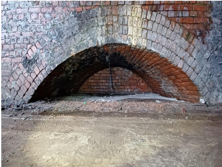
Photo 33: Open joints up to 20mm deep with friable mortar, wet brickwork, hollow sounding brickwork to crown of arch barrel and surface spalling to face ring of 2 nd relieving arch from south end of central pier west face.
