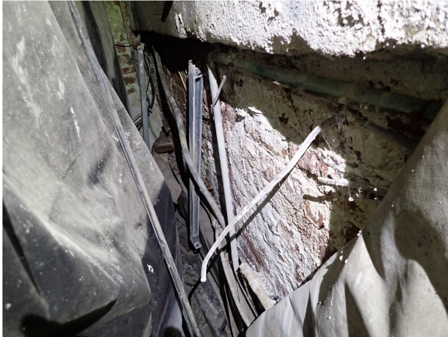
Photo 45: Wet brickwork and water pooling at base of east abutment at exposed section below Photo. 37.
