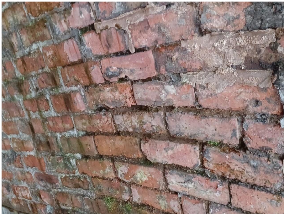
Photo 16: Area of wet friable mortar and open joints 1100x2000x15mm to quarter point at northwest end of span 1 arch barrel.
