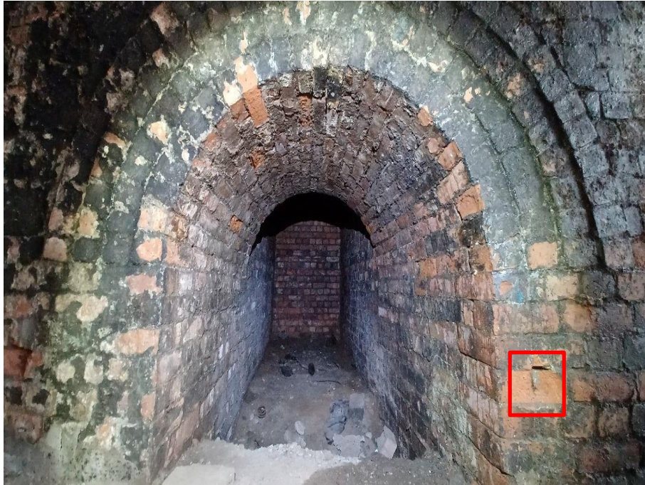
Photo 25: Open joints up to 30mm deep, wet friable mortar, surface spalling, and leachate staining to arch barrel and exposed re-bar to face ring of 3 rd relieving arch from south end of west abutment span 1.
