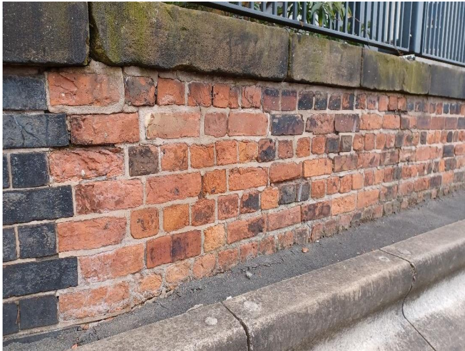
Photo 67: Isolated open joints and surface spalling to brickwork of north parapet south face.
