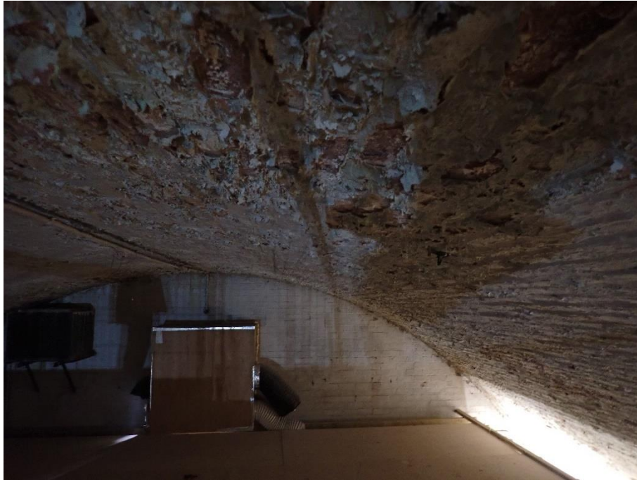
Photo 41: Hollow sounding area of brickwork 3x1.5m to west quarter point starting at south infill wall with 10mm displaced course of bricks within same area of span 2 arch barrel.
