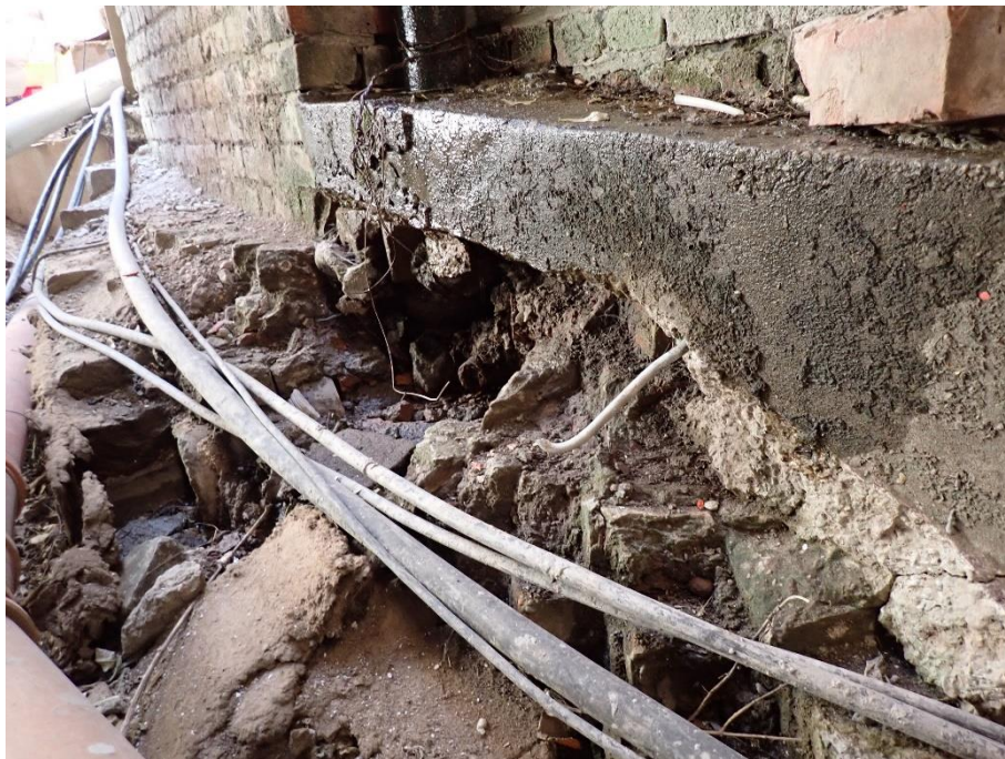
Photo 42: Area of section loss 1100x200x110mm to concrete section at base of east abutment north end.
