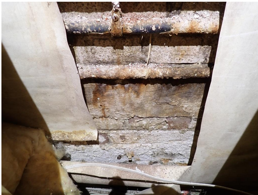
Photo 46: Staining to exposed section of east abutment at approx. mid-span.
