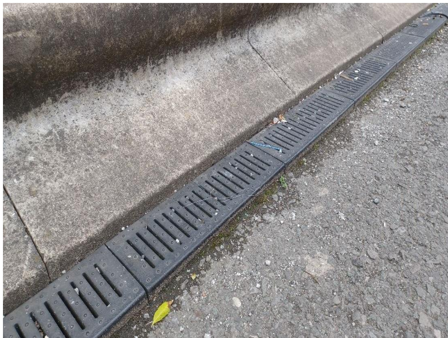
Photo 64: Gutter raised above carriageway surfacing by 30mm affecting drainage.
