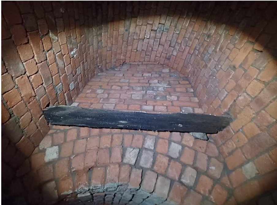
Photo 23: Wet friable mortar and damp brickwork to west face of 1 st relieving arch from south end of west abutment span 1.
