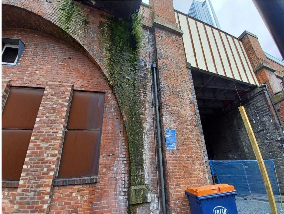
Photo 53: Moss/vegetation growth, isolated surface spalling, isolated open joints, and water ingress (wet) to east spandrel of span 2 south elevation below footbridge.
