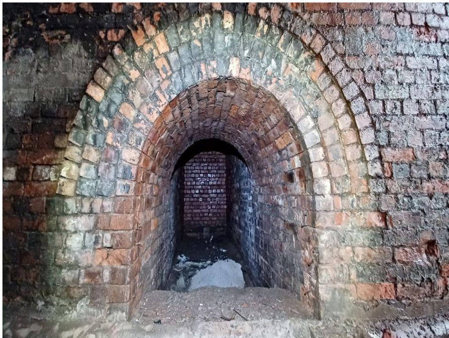
Photo 26: Open joints up to 30mm deep, wet friable mortar, surface spalling, and leachate staining to arch barrel of 4 th relieving arch from south end of west abutment span 1.
