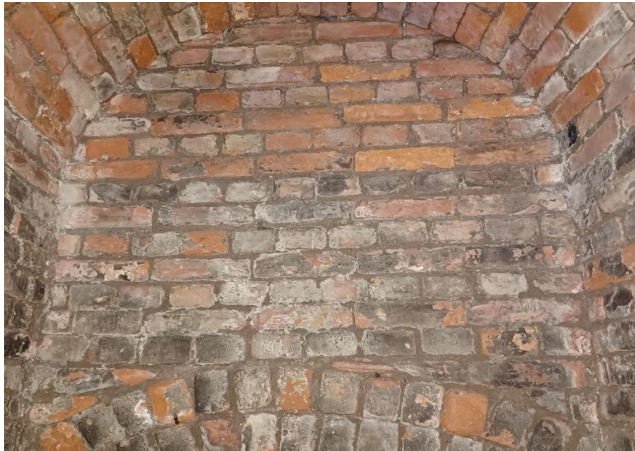
Photo 29: Wet friable water and drummy brickwork to west face of 5 th relieving arch from south end of west abutment span 1.
