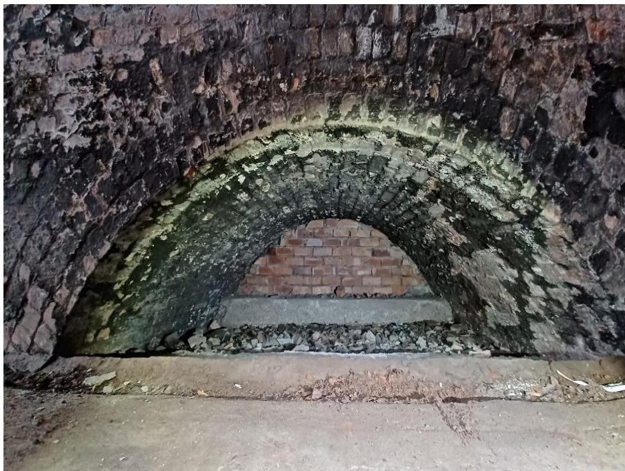
Photo 32: Moss growth and leachate deposits to arch barrel and face ring of 1 st relieving arch from south end of central pier west face.
