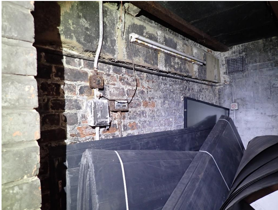
Photo 47: Isolated surface spalling and staining to brickwork at south end of east abutment.
