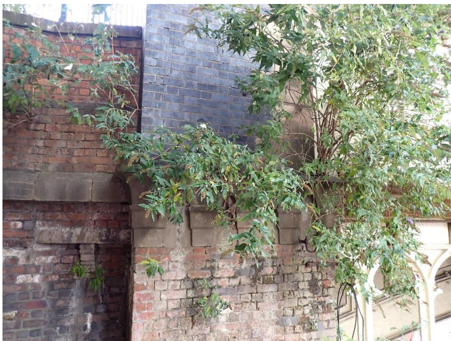
Photo 56: Vegetation growth to top section of west abutment north end.
