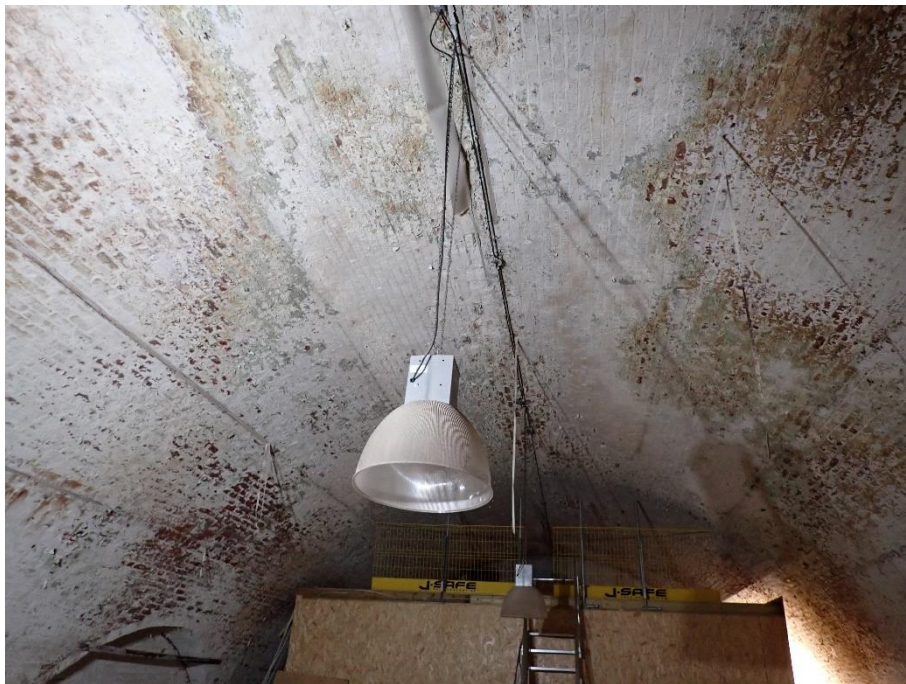
Photo 36: Typical paintwork breakdown throughout to internal section of span 2 soffit.
