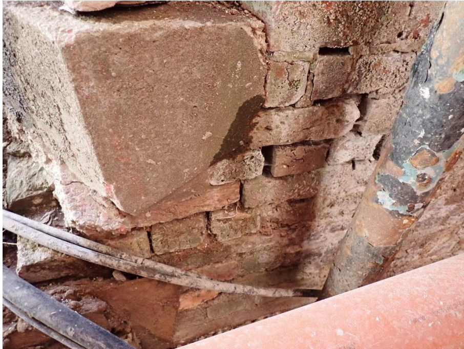
Photo 43: Area of displaced brickwork and mortar loss 500x250mm to north end of east abutment.
