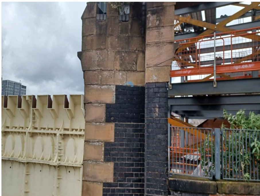
Photo 68: Isolated open joints and vegetation growth to northwest pilaster.
