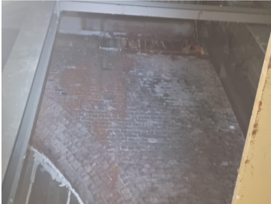
Photo 51: Leachate staining to east spandrel of span 1 south elevation.
