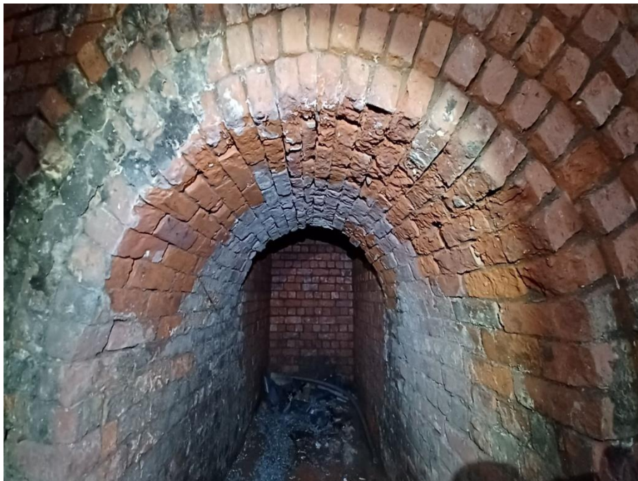
Photo 22: Open joints up to 30mm deep, wet friable mortar, surface spalling, and leachate staining to arch barrel of 1 st relieving arch from south end of west abutment span 1.
