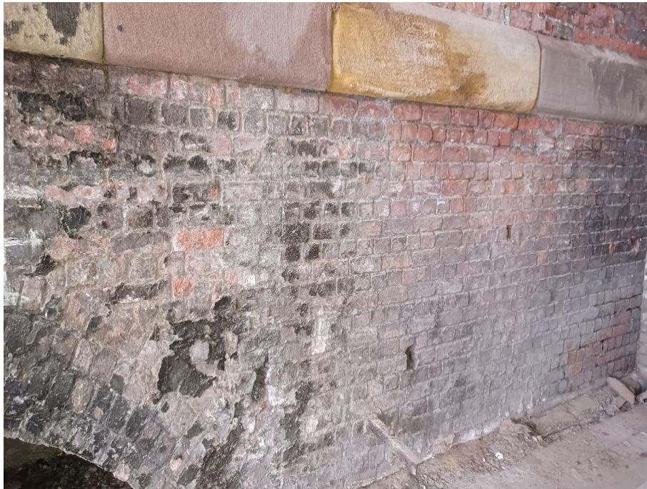
Photo 31: 2 No. missing bricks and leachate staining to south end of central pier west face.
