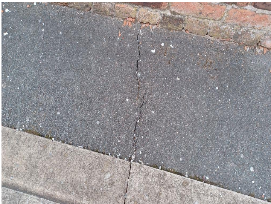
Photo 66: Cracks in footway surfacing adjacent to north parapet.
