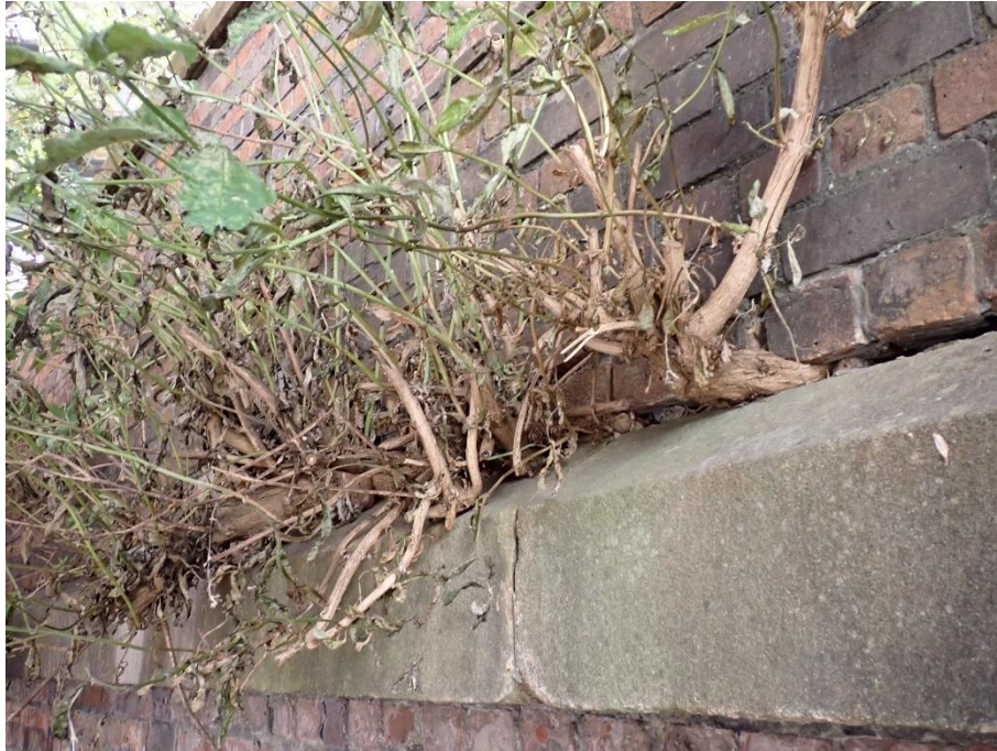
Photo 57: Significant root growth displacing brickwork up to 20mm to string course of north elevation of span 1.
