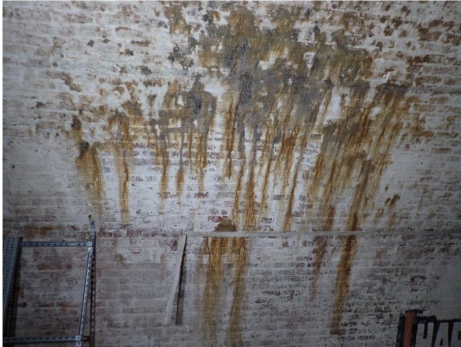
Photo 37: Calcite staining and active water ingress (dripping) to northeast end to internal section of span 2 soffit.
