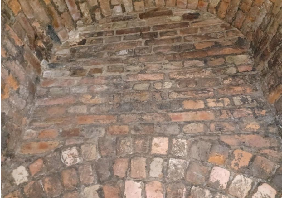
Photo 27: Wet friable water to west face of 4 th relieving arch from south end of west abutment span 1.
