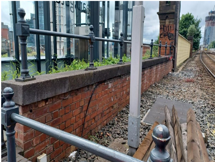
Photo 62: Isolated open joints, joint fractures, leachate staining, surface spalling, and minor vegetation growth to north face of south parapet.
