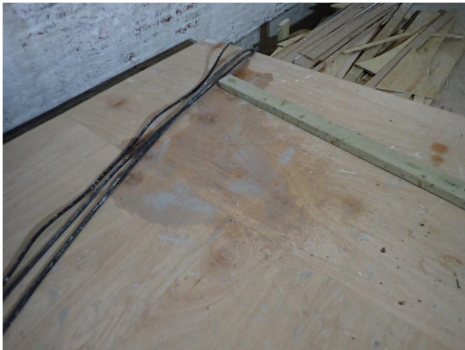
Photo 38: Water pooling to temporary ceiling below water ingress in previous photograph.
