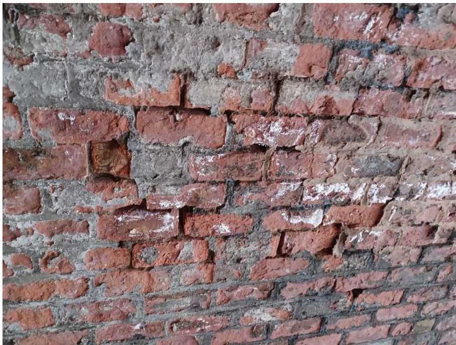
Photo 14: Area of spalling and open joints 1m 2 x30mm at mid-span of west face of span 1 arch barrel.
