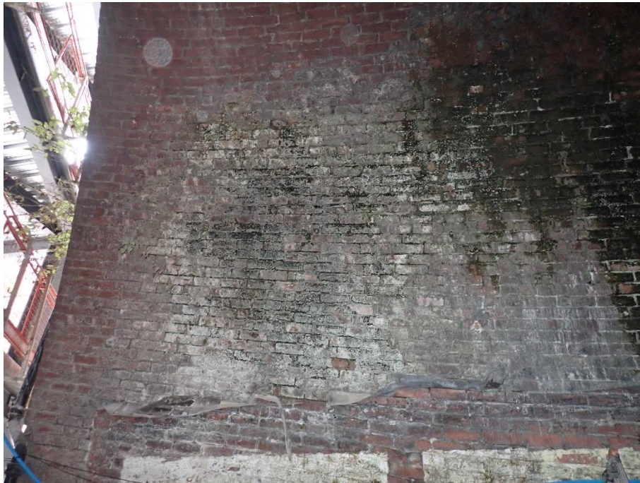
Photo 35: Leachate staining, open joints 10-15mm deep, and hollow sounding area of brickwork 3000x5000mm to northeast of span 2 arch barrel.
