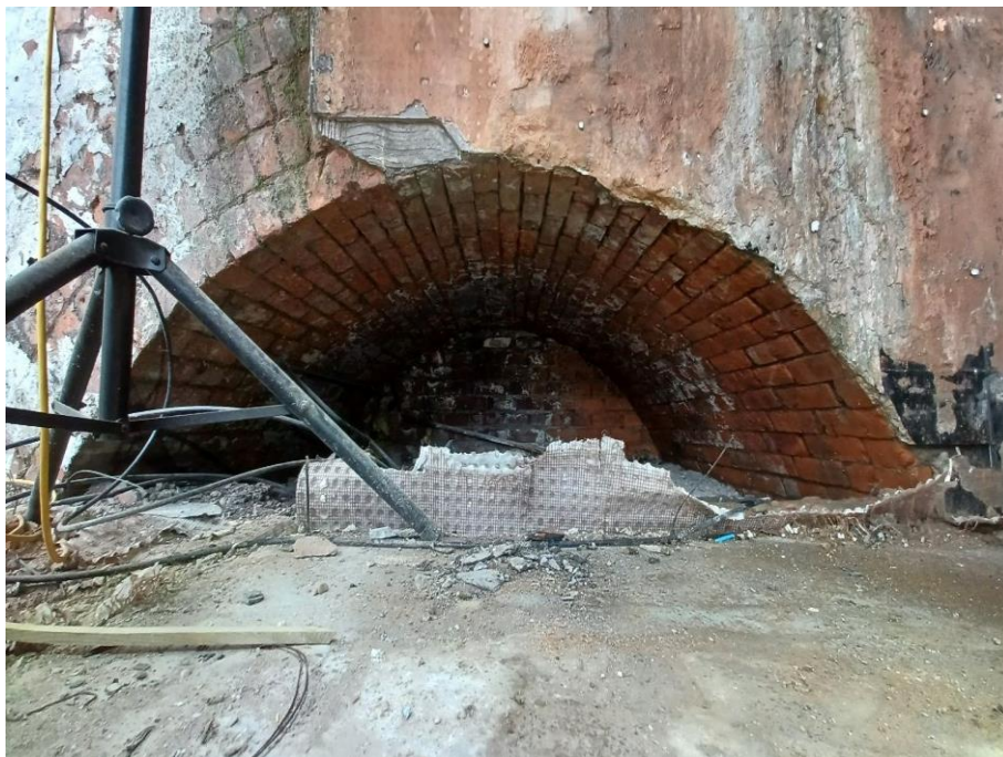
Photo 34: Wet brickwork and friable mortar to 3 rd relieving arch from south end of central pier west face.
