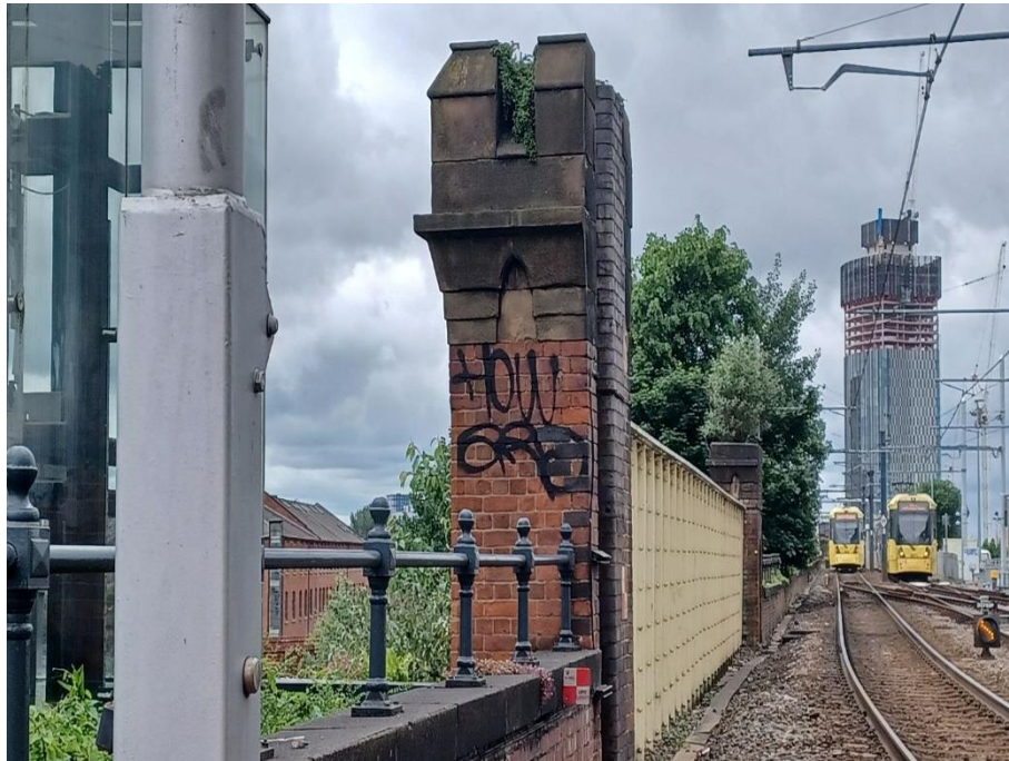
Photo 63: Vegetation and graffiti to southwest pilaster.
