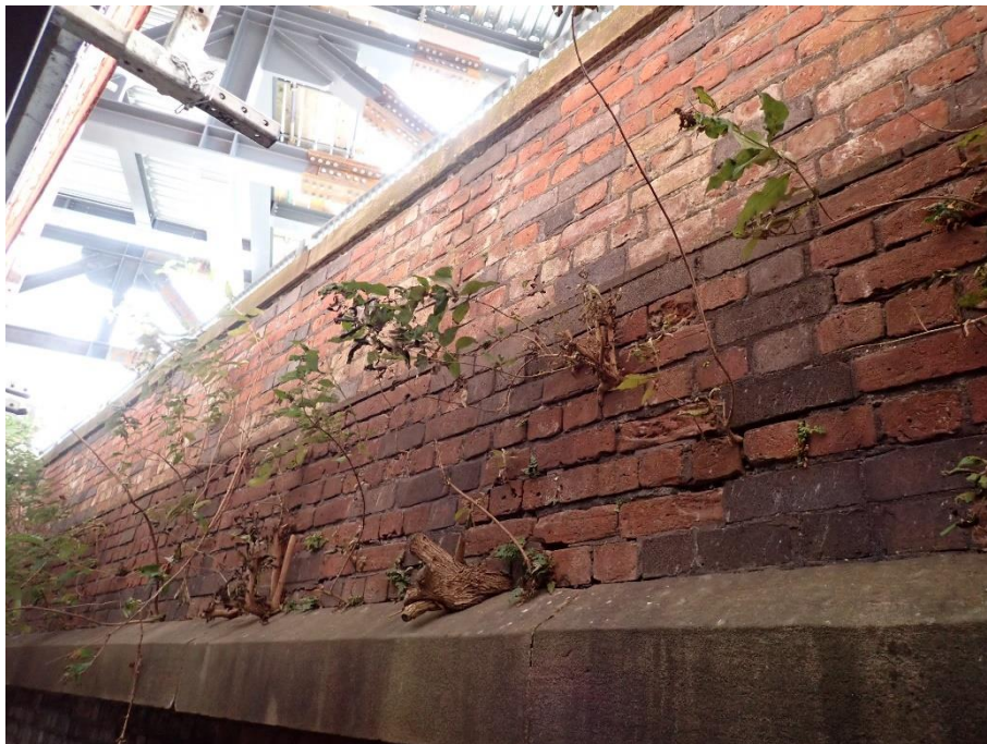
Photo 58: Typical vegetation growth and isolated surface spalling to brickwork of north elevation parapet.
