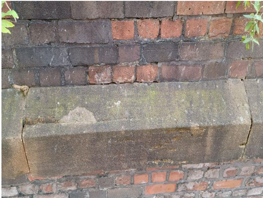
Photo 59: Horizontal hairline fracture to string course stone between span 1 & 2 of north elevation.
