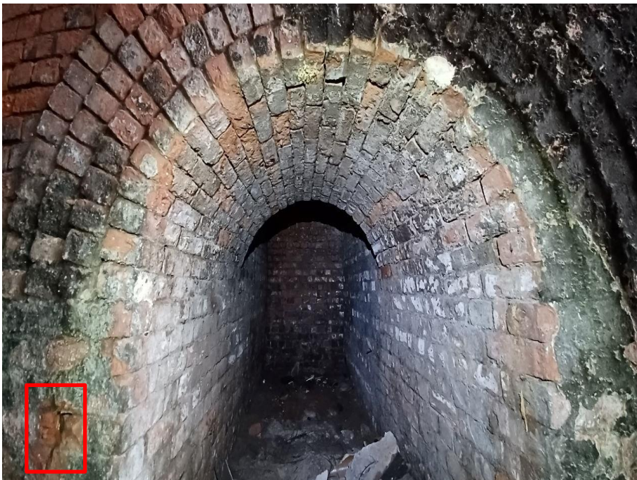
Photo 24: Open joints up to 30mm deep, wet friable mortar, surface spalling, and leachate staining to arch barrel and exposed re-bar to face ring of 2 nd relieving arch from south end of west abutment span 1.
