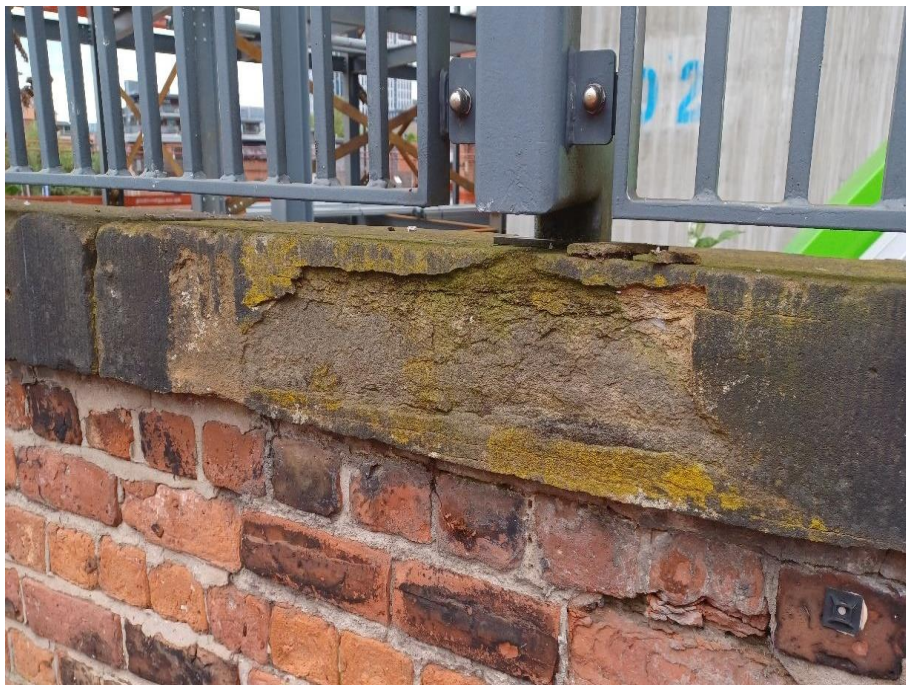
Photo 70: Surface spall to coping stone at mid-span of north parapet south face.
