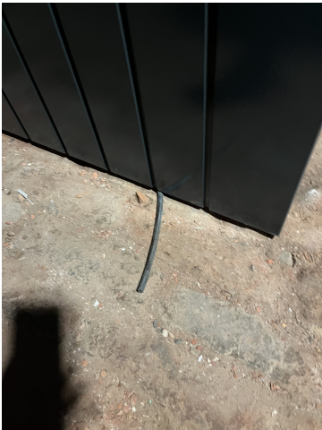
Causing intumescent seal to drag and pull out of newly installed fire door.
