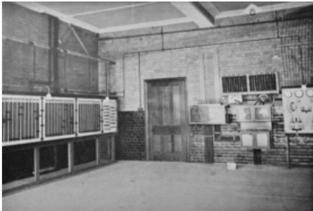
2.3.7 Switchboard (ground floor), 1906
