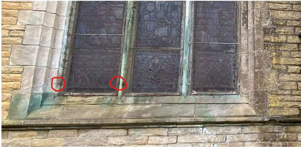
Fig 11 Ferrous fixing clamps used to secure metal security grilles
