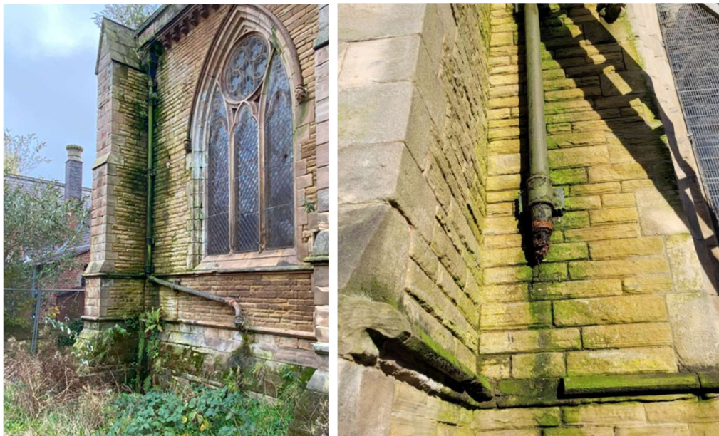
Fig 2 & 3 Damp and vegetation growth associated with corroding cast iron pipes in 2024
