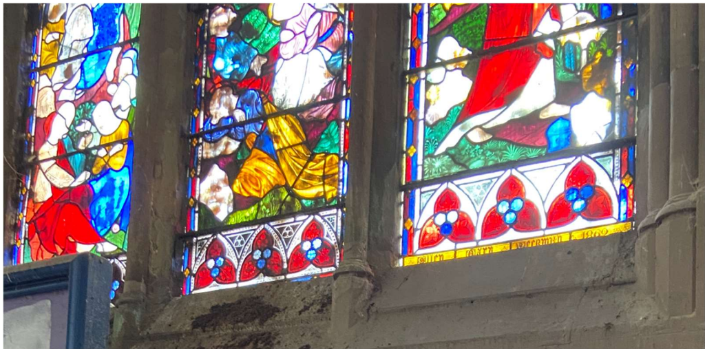
Fig 16 missing pieces within stained-glass panels
