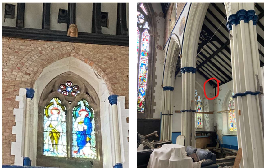
Fig 41 and 42 cut felt to upper roof and missing ends to trusses
