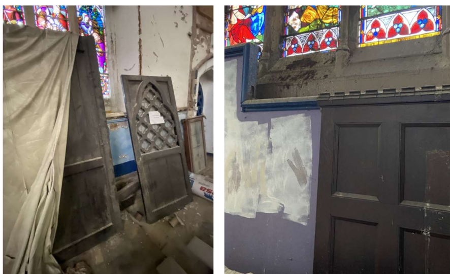
Fig 37 & 38 loose timber screen and painted panelling beneath window
