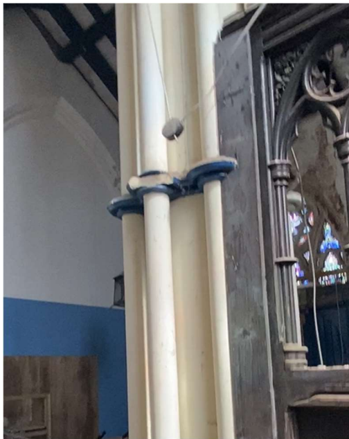
Fig 32 Broken collar feature to the fluted column
