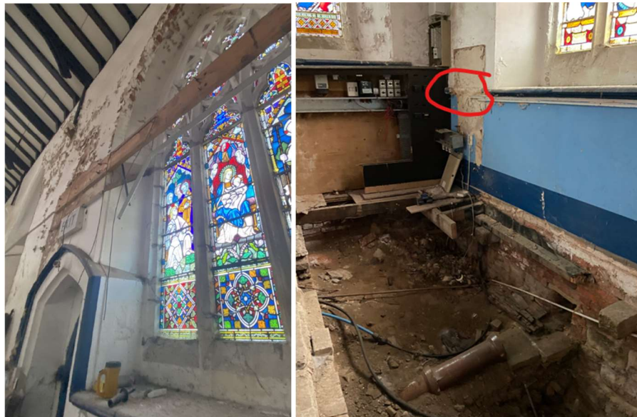
Fig 33 & 34 Blue painted plaster moulding to window cills and door surrounds including some missing sections
