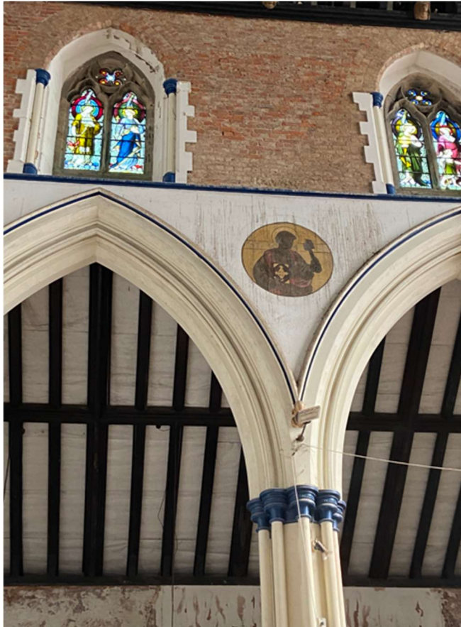
Fig 35 Plaster previously removed from clerestorey, damaged plaster to the external wall in background, plastered partition with decorative roundel
