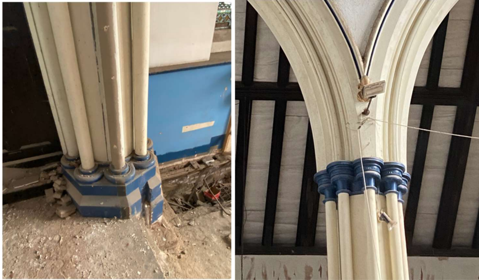
Fig 30 & 31 Former partition where plinth is incomplete and services fixed to columns
