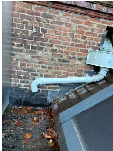
New Hopper & downpipe
