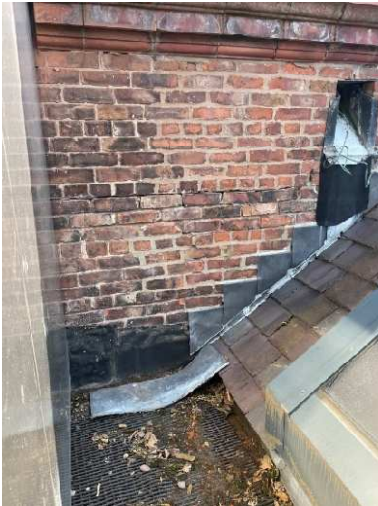
Downpipe & hopper missing
