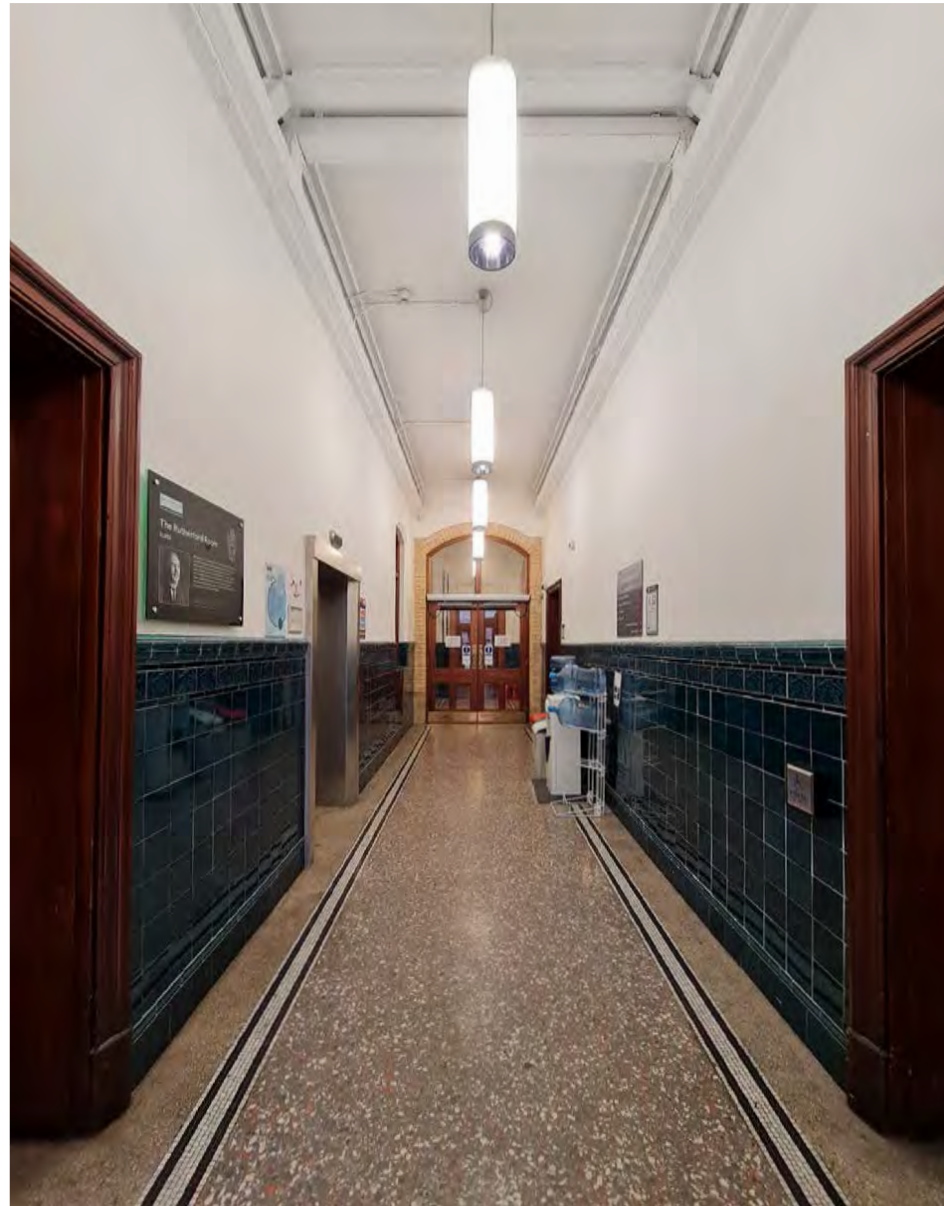
▲ High Level Trunking in Corridor to be Removed to Reveal Historic Ceiling
