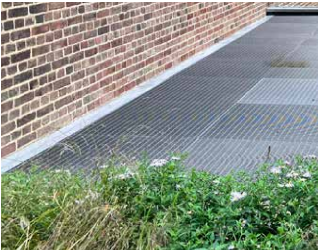
Galvanised steel ventilation grilles set within planted areas to mitigate visual impact
