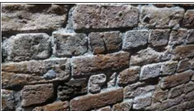
Spalling Brickwork in Basement
