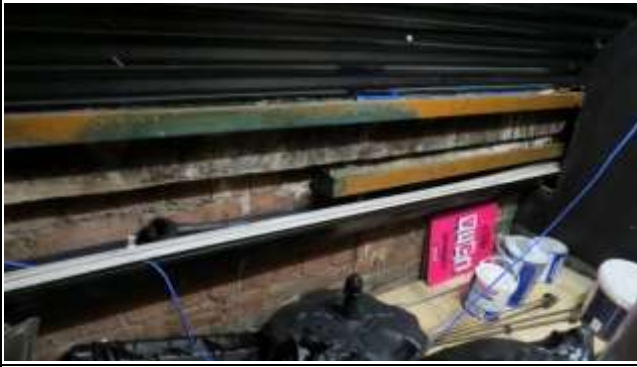
Supplementary Guttering and Ceiling Lining
