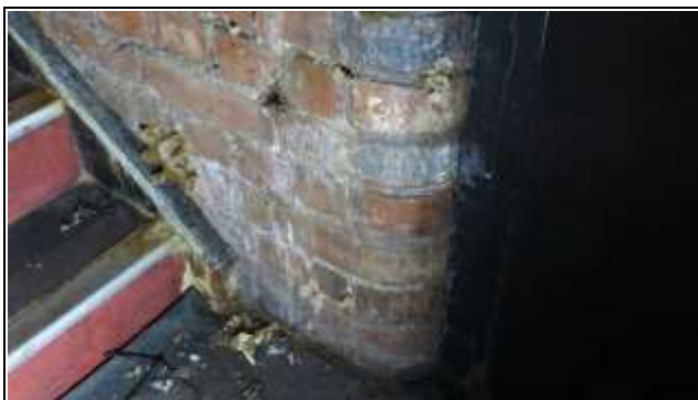
Dry Rot on Rear Staircase
