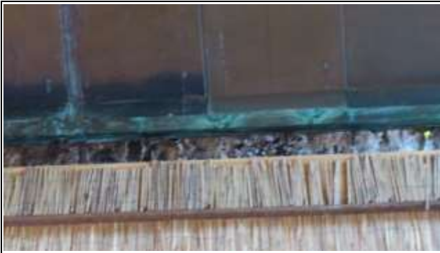
Evidence of Overflowing Gutters
