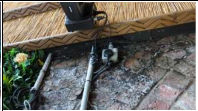
Impact of Water Ingress on Brickwork
