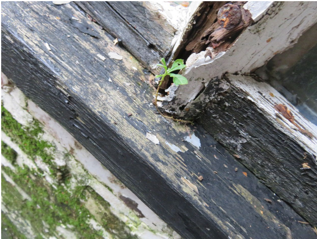
Rotten window to W9.
