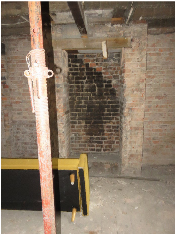
Retain, reassess and re-plaster.
