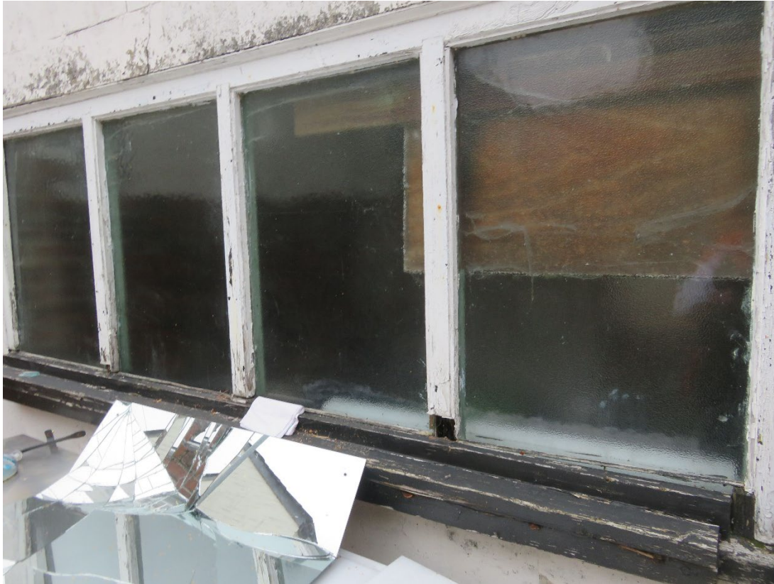
Rotten window to W8.
