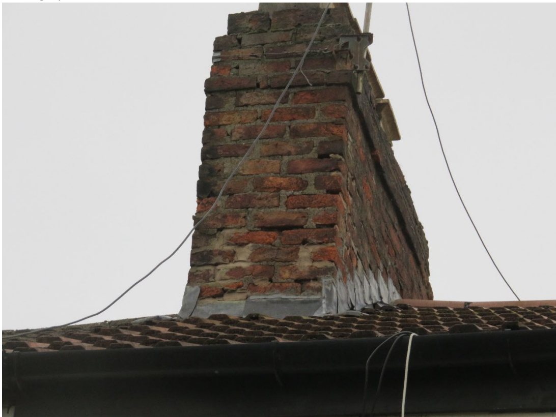
Carry out patch pointing in lime based mortar to stack, do not rebuild.
