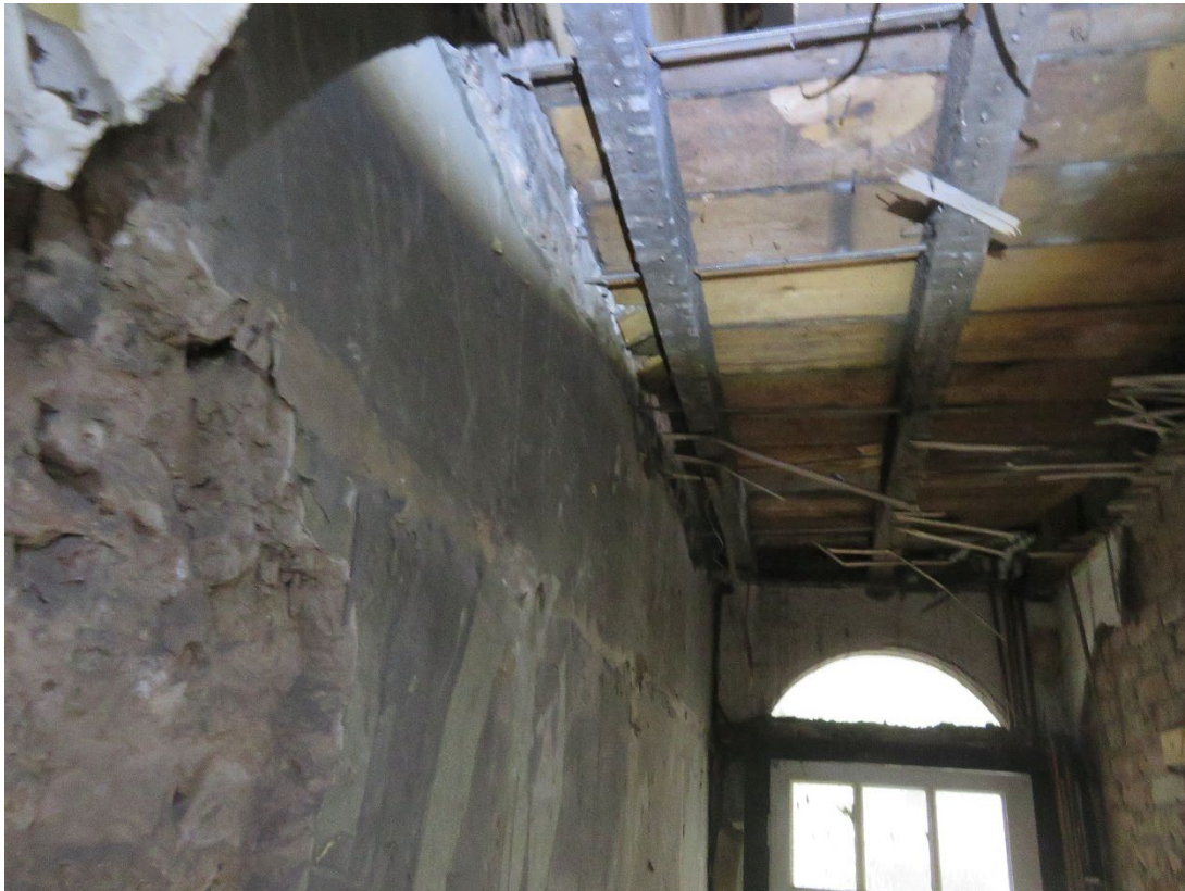
Ineffective lateral restraint in hallway.
