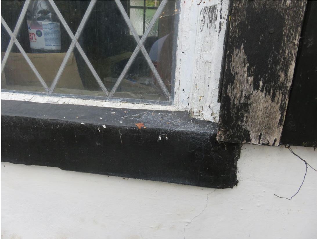
Wet rot to W1.
