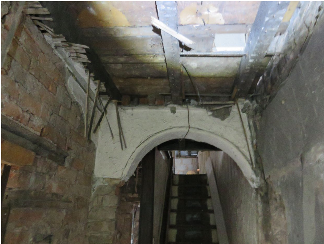
Ineffective thread in stainless steel bars not retaining gable wall.
