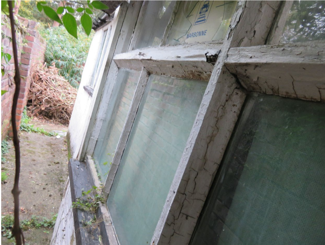
Rotten window to W9.
