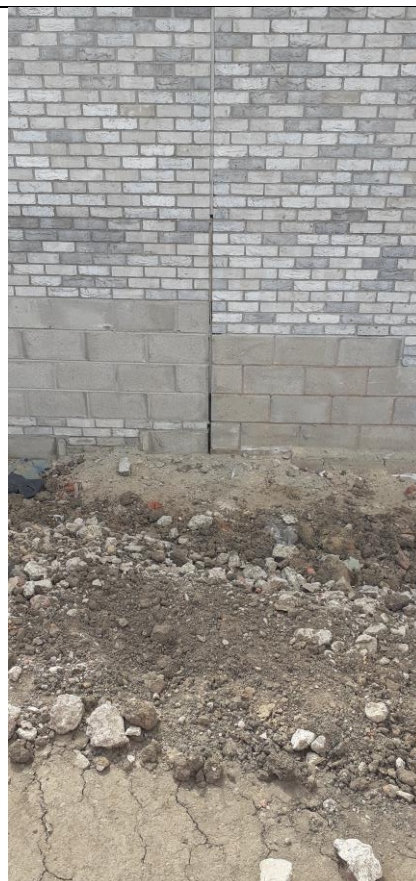
Backfilling to boundary wall – NT02 Joint in wall not filled
