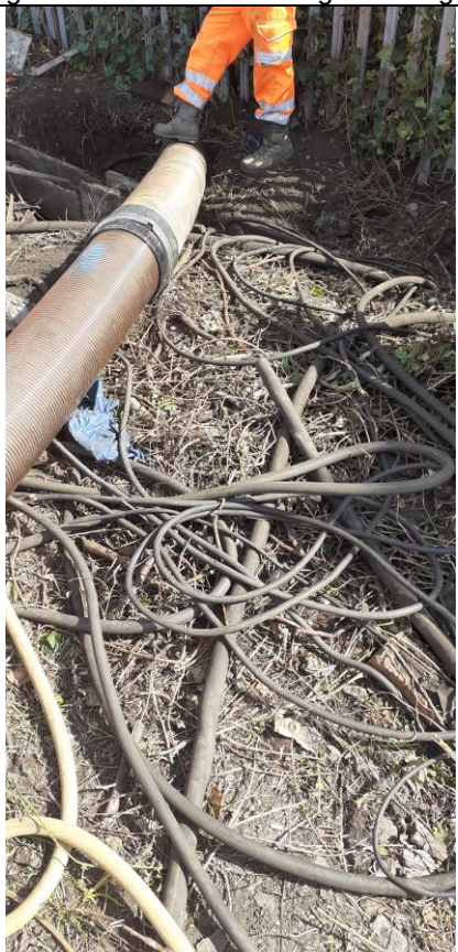
Numerous dead cables exposed and removed adjacent railway boundary
