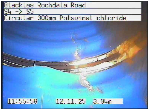
1, 00:00:39, 3.93 m Deformed sewer or drain, 5%
