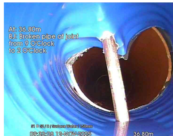
8, 00:02:46, 36.80 m Broken pipe at joint from 9 o'clock to 2 o'clock
