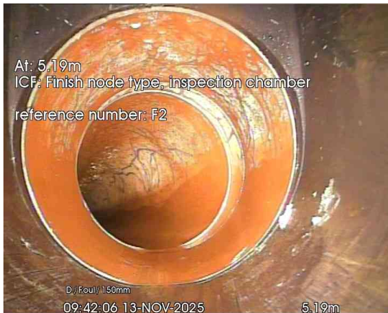
1, 00:00:18, 5.19 m Finish node, inspection chamber, reference: F2
