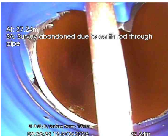
11, 00:03:42, 37.24 m Survey abandoned, due to earth rod through pipe
