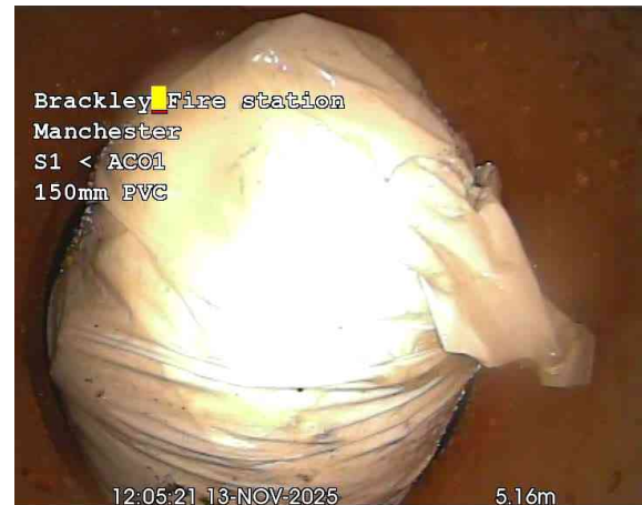
2, 00:00:24, 5.16 m Survey abandoned, ACO outlet bagged off
