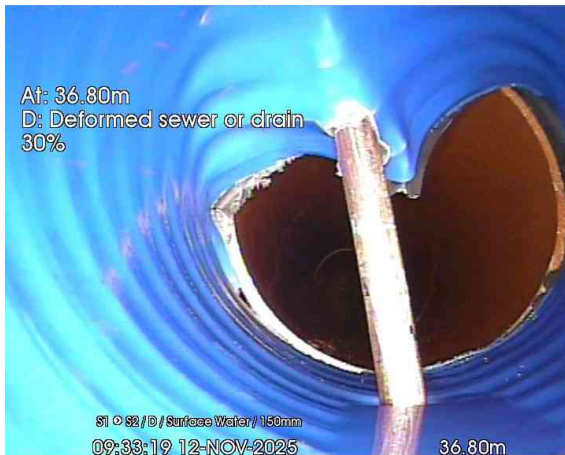
9, 00:02:47, 36.80 m Deformed sewer or drain, 30%
