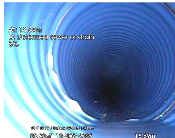
4, 00:01:25, 18.69 m Deformed sewer or drain, 5%
