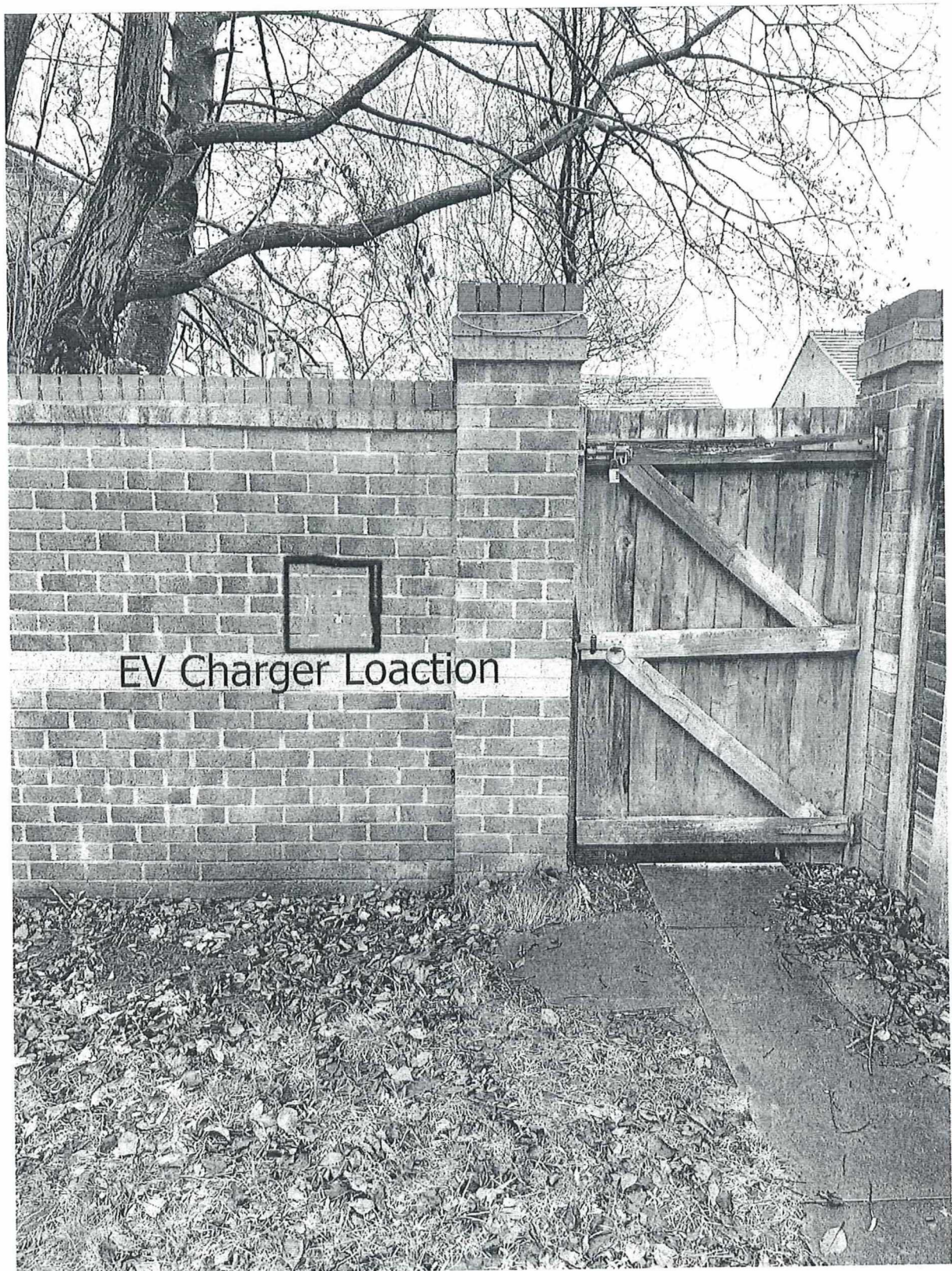
Photo 1: This shows the location (in purple colour) of the Ohme EV charger inside the garden wall.
