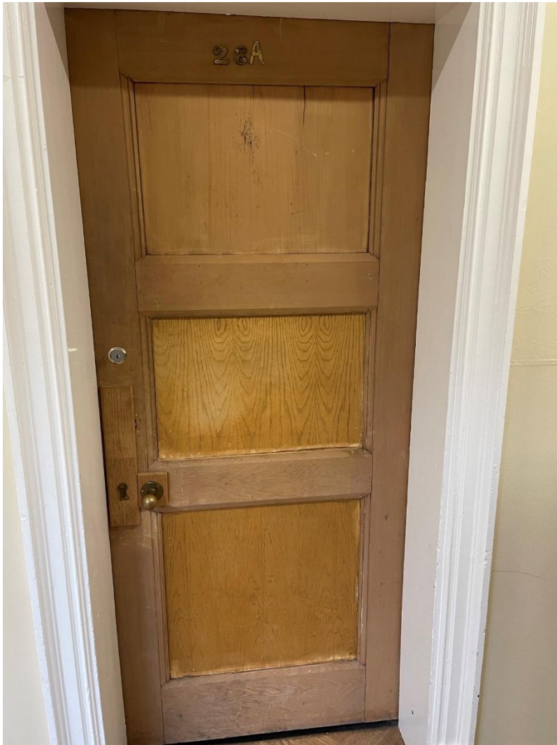
Photo 5. Example of timber fire resistant door to be repaired and coated with Envirograf.
