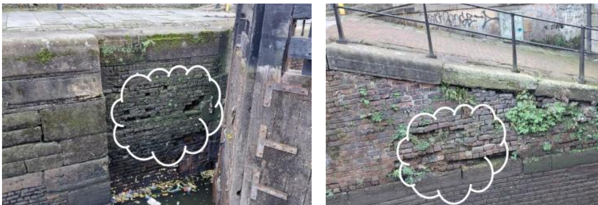
Figure 2 – Evidence of spalling brickwork
