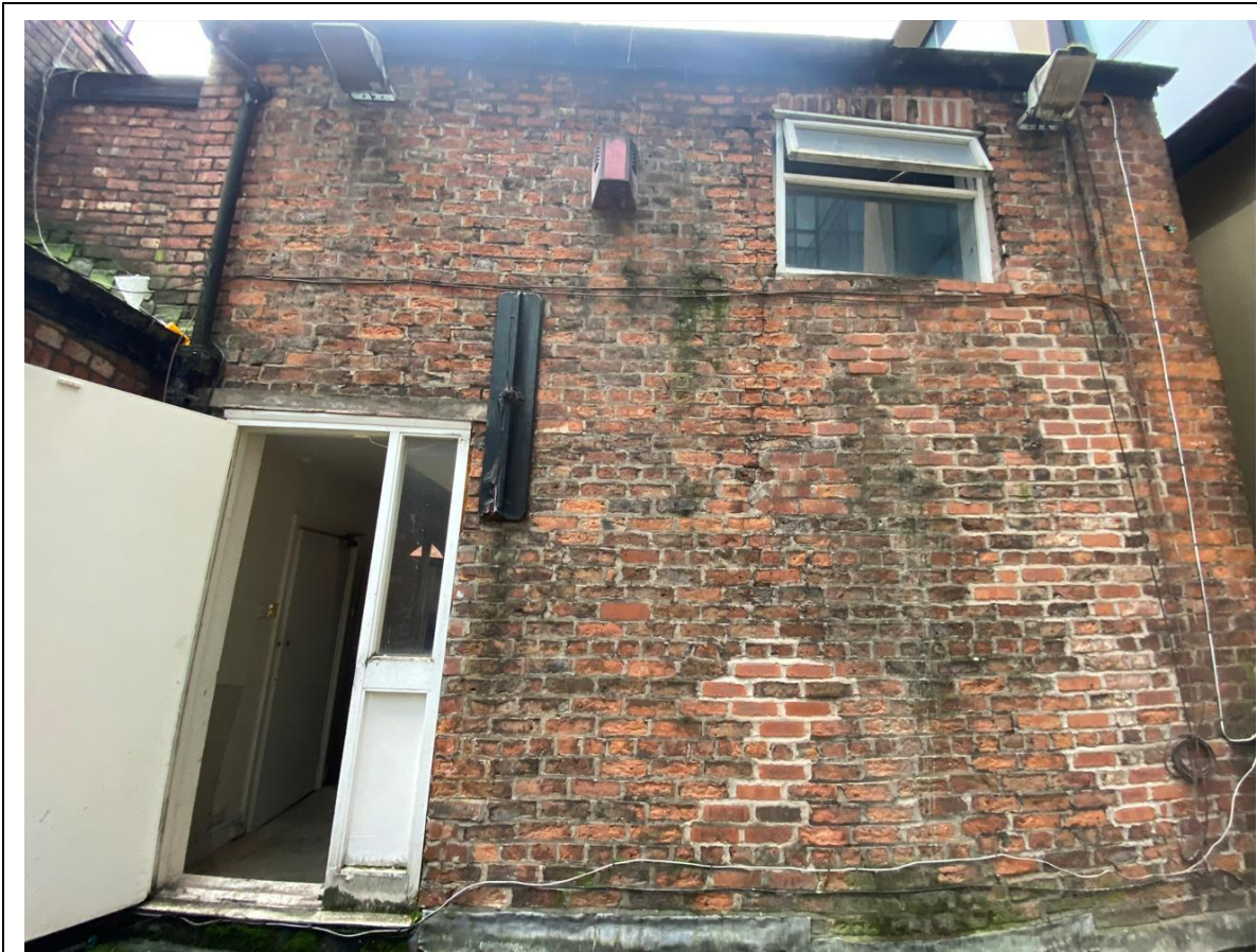
^ North elevation – west side first and second floor. This c.1820s elevation contains a modern doorway and window. The brickwork is in poor condition and has been repointed in cement and had areas of brick replacement.
