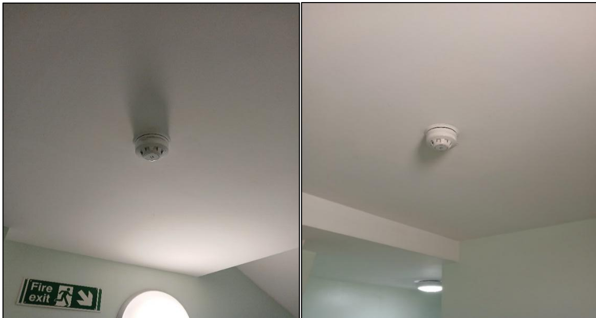
Figure 9 – Smoke detectors installed in the communal corridors and the staircase.
