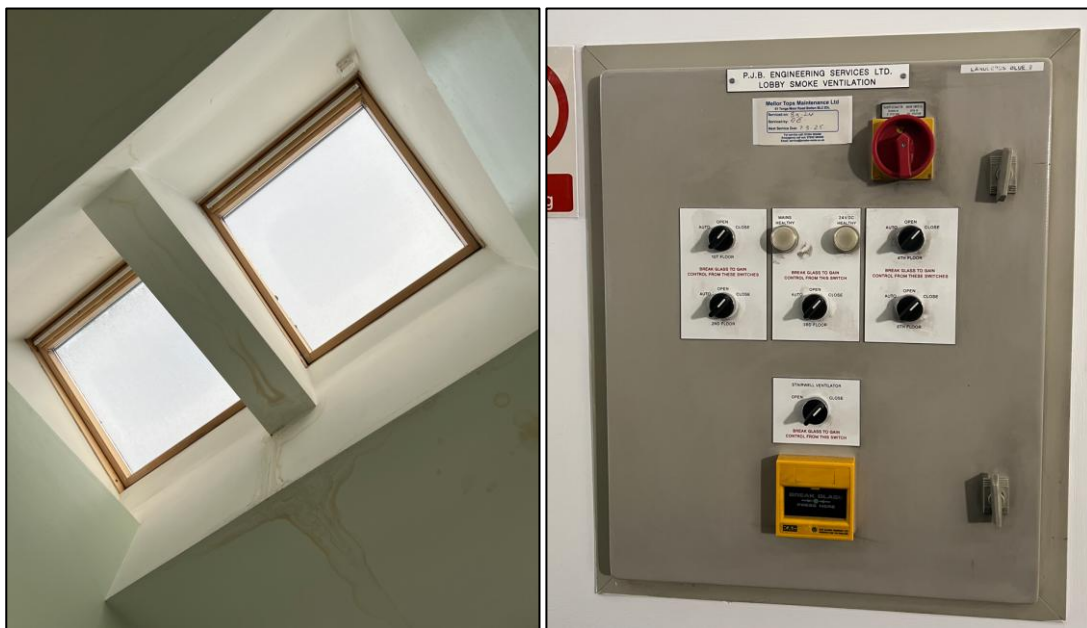
Figure 7 – AOV's at the head of the staircase (left); and lobby smoke ventilation on the ground level (right), image taken by Octa Fire.
