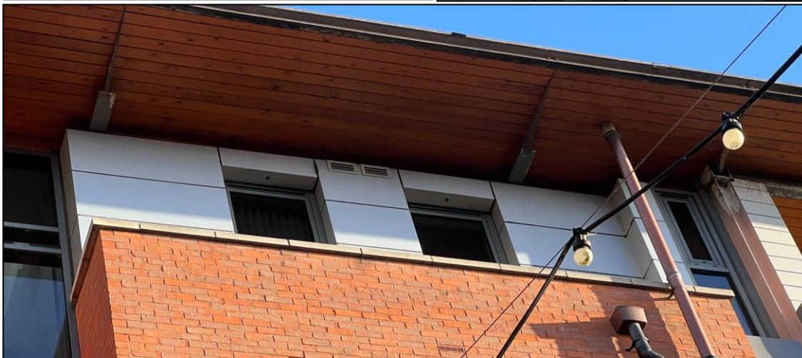
Figure 15 – Silver ACM cladding panels – EWT4.
