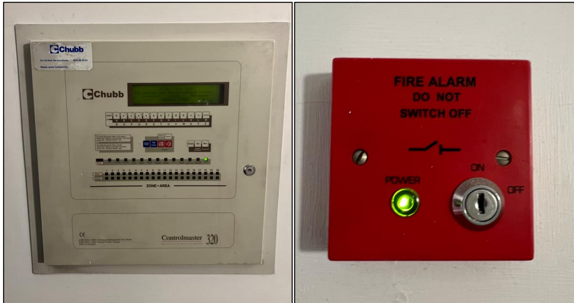
Figure 8 – Fire alarm, image taken by Octa Fire.
