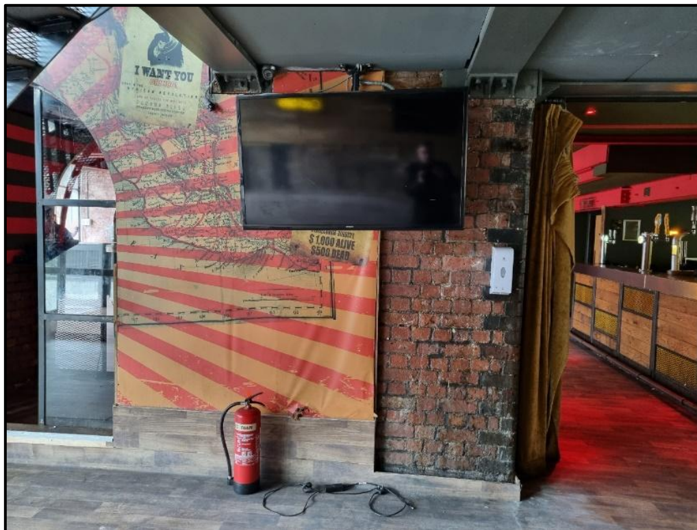
Images showing some of the damage caused by water ingress.
