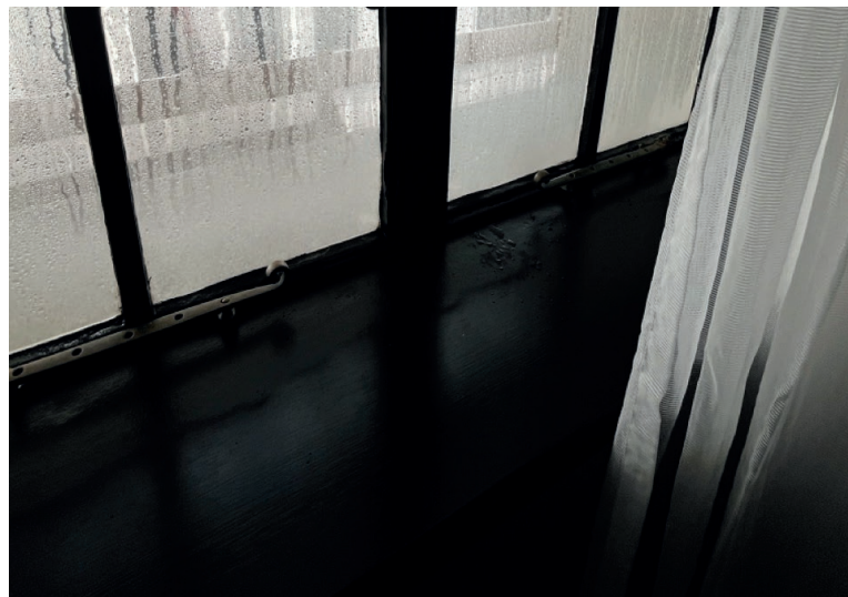
Image above: Example of cill with water damage.
