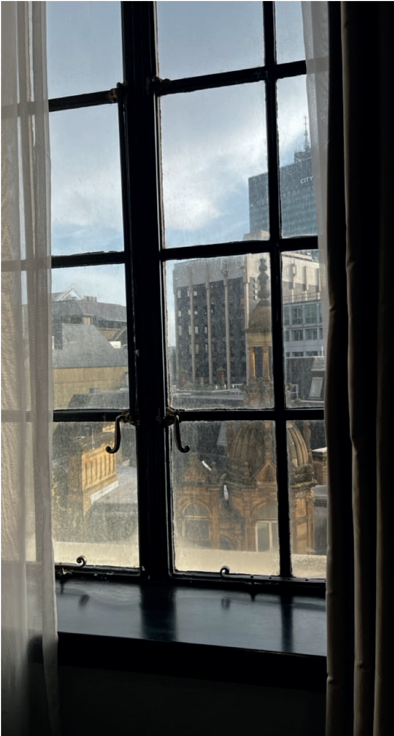
Image: Example window set with deep reveal with not-original cill showing signs of water damage.
