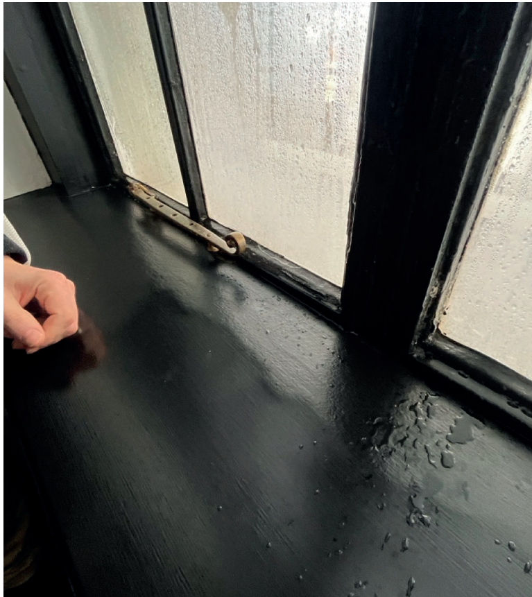
Image: Example window set with deep reveal with non-original cill showing signs of water damage as a result of excessive condensation.
