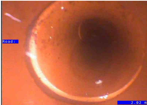
SVP4X_66a6968e-d7a4-4fe5-8506-9ba4780cf1a8_20251203_134551_244.jpg, 00:00:20, 2.02 m Joint displaced, medium (between 1.0 and 1.5 times the pipe wall thickness), 4 o'clock to 12 o'clock
