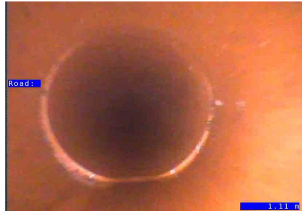
L1X_49b09f59-0a70-4085-be3e-0f0e73be2d4a_20251203_103502_780.jpg, 00:00:22, 1.11 m Joint displaced, medium (between 1.0 and 1.5 times the pipe wall thickness), 12o'clock to 12o'clock - holding small amount of water
