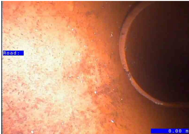
L1X_91cd0ffd-4aeb-4ee4-8e12-1b3fc78f620e_20251203_103355_573.jpg, 00:00:11, 0.00 m Joint displaced, medium (between 1.0 and 1.5 times the pipe wall thickness), 12o'clock to 12o'clock
