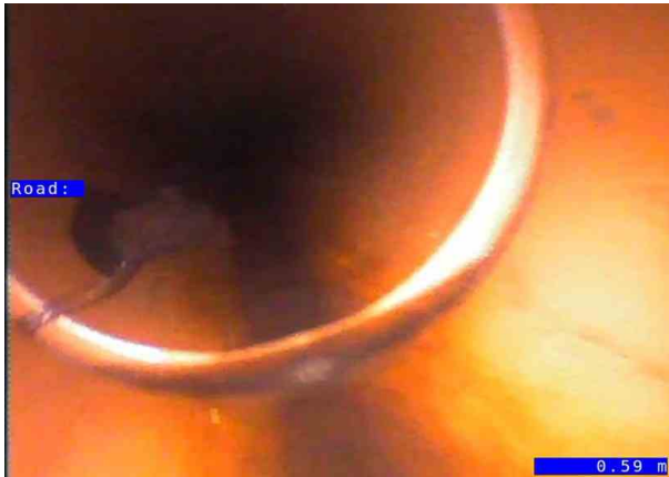
RGY3X_fa14638b-8e7b-4073-b8aa-469931047013_20251203_153922_867.jpg, 00:00:07, 0.60 m Joint displaced, medium (between 1.0 and 1.5 times the pipe wall thickness), 12o'clock to 12o'clock
