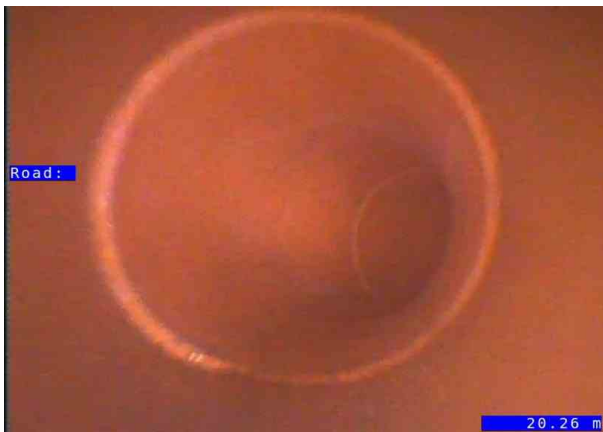
U_SX_9328f0eb-69a5-490c-afde-69c3e01f9e95_20251203_104849_191.jpg, 00:01:49, 20.26 m Joint displaced, medium (between 1.0 and 1.5 times the pipe wall thickness), 12 o'clock to 12 o'clock
