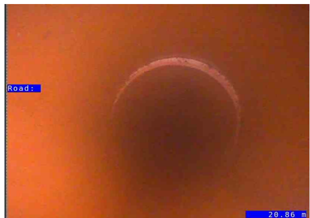
L1X_f99854c1-b0e6-47cd-af4f-85c6c2cadd68_20251203_101730_713.jpg, 00:03:58, 20.90 m Joint displaced, medium (between 1.0 and 1.5 times the pipe wall thickness), 100'clock to 30'clock
