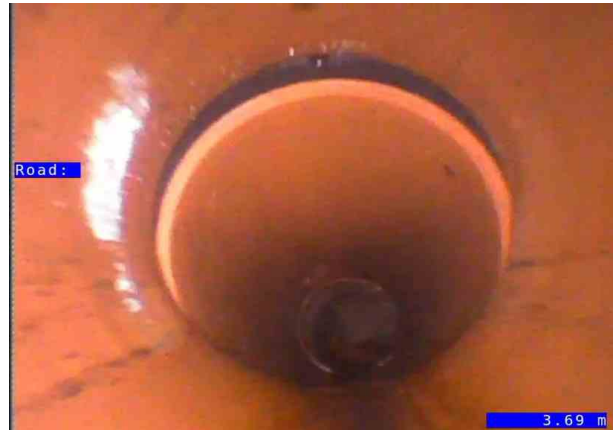
RGY3X_b3cc2459-c923-4239-9af6-311d4437dfce_20251203_154005_866.jpg, 00:00:18, 3.70 m Joint displaced, medium (between 1.0 and 1.5 times the pipe wall thickness), 8o'clock to 3o'clock
