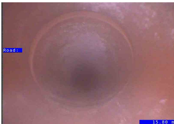
L2X_4f31c3a5-ae38-4c2a-a94d-4b54eaf4b7cc_20251202_112430_173.jpg, 00:02:03, 15.80 m Joint displaced, medium (between 1.0 and 1.5 times the pipe wall thickness), 8 o'clock to 2 o'clock
