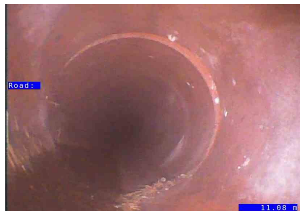
U_SX_536b1336-2e10-4062-bdfd-c81599bc85a0_20251203_104624_873.jpg, 00:00:58, 11.08 m Roots, mass
