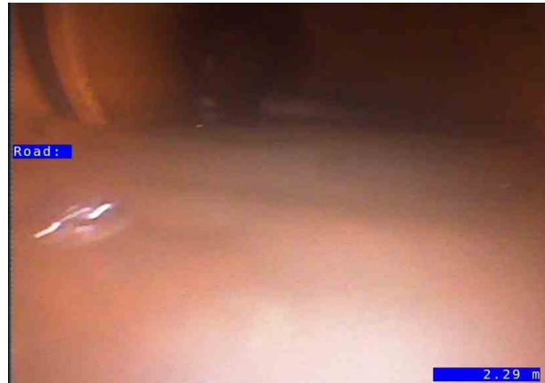
SVP4X_d5950e44-b5b1-41be-ab3b-8ed712a09bb0_20251203_134714_243.jpg, 00:00:21, 2.30 m Joint displaced, medium (between 1.0 and 1.5 times the pipe wall thickness), 12 o'clock to 12 o'clock - holding water
