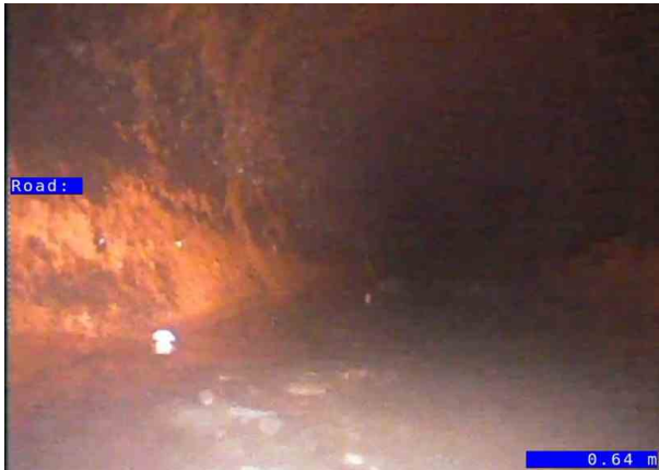
MH1X_820c11f4-37fe-4bd5-b413-ada0139f7de8_20251202_1 05344_487.jpg, 00:00:18, 0.65 m Debris, other, start, Along bottom of pipe
