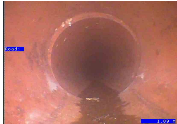
U_SX_1315d83b-f9db-4ddf-9afc-24fe433f1d7b_20251203_104456_834.jpg, 00:00:17, 1.09 m Joint displaced, medium (between 1.0 and 1.5 times the pipe wall thickness), 9 o'clock to 2 o'clock
