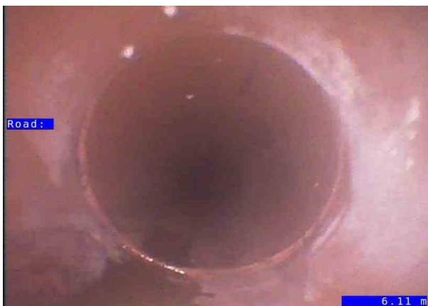
U_SX_9ef3008b-2c02-4a29-81b4-5271e2ca8f5d_20251203_104541_449.jpg, 00:00:38, 6.11 m Joint displaced, medium (between 1.0 and 1.5 times the pipe wall thickness), 4 o'clock to 9 o'clock
