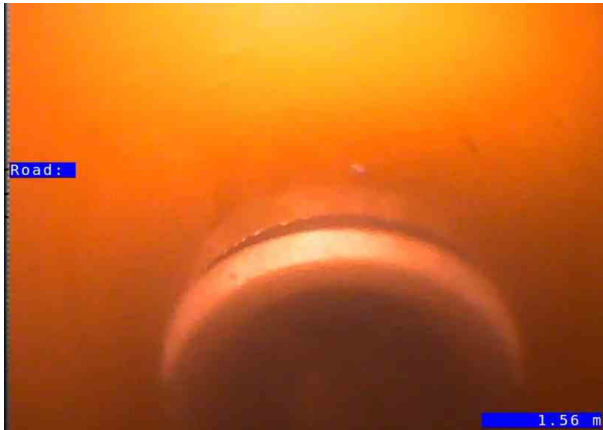
SVP3X_9a0b19a9-f58c-4638-9b3e-c137b5c45634_20251203_134912_322.jpg, 00:00:23, 1.56 m Joint displaced, large (over 1.5 times the pipe wall tickness), 9o'clock to 3o'clock
