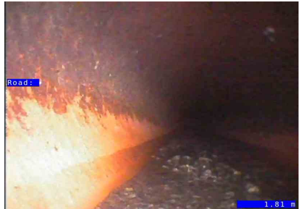
MH1X_cb103d0c-5897-421a-9b4a-da42e4a442c3_20251202_105156_201.jpg, 00:00:24, 0.10 m Debris, other, start, Along the bottom of the pipe
