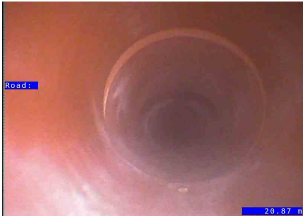
L2X_6217cadd-cb9a-4392-b23f-86bce4c8741d_20251202_112528_043.jpg, 00:02:44, 20.87 m Joint displaced, medium (between 1.0 and 1.5 times the pipe wall thickness), 9 o'clock to 2 o'clock
