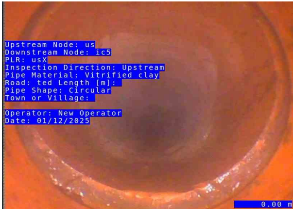
U_SX_d2b81afc-145b-409c-b27d-2755f2851e11_20251203_104420_930.jpg, 00:00:01, 0.00 m Joint displaced, large (over 1.5 times the pipe wall thickness), 12 o'clock to 12 o'clock
