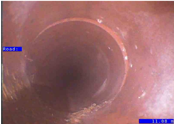
U_SX_ee523dcc-4451-43ba-9b95-2b1b84c7e0c2_20251203_104645_232.jpg, 00:00:58, 11.10 m Joint displaced, medium (between 1.0 and 1.5 times the pipe wall thickness), 9 o'clock to 1 o'clock
