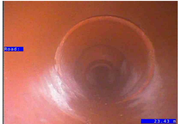
L2X_bbc57da1-e6b6-4a01-a7d8-016d5efe7e10_20251202_112556_754.jpg, 00:03:03, 23.45 m Joint displaced, medium (between 1.0 and 1.5 times the pipe wall thickness), 9 o'clock to 5 o'clock
