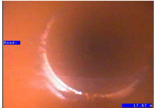
L1X_721125ff-d591-4ad2-95dd-fe3bc46f417e_20251203_101449_985.jpg, 00:03:45, 17.87 m Joint displaced, medium (between 1.0 and 1.5 times the pipe wall thickness), 30'clock to 90'clock
