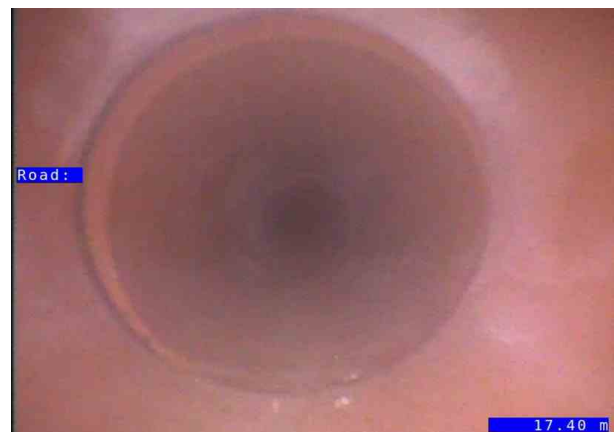
L2X_e70af9f8-0e39-4ae4-8797-9795091f6584_20251202_112458_731.jpg, 00:02:18, 17.40 m Joint displaced, medium (between 1.0 and 1.5 times the pipe wall thickness), 7 o'clock to 2 o'clock
