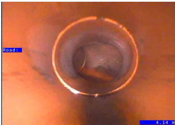
RGY3X_446cb528-bb39-4c6f-bd47-20cc33bca0bf_20251203_154050_634.jpg, 00:00:19, 4.15 m Joint displaced, medium (between 1.0 and 1.5 times the pipe wall thickness), 12o'clock to 12o'clock
