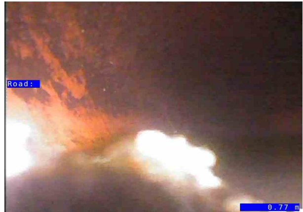
MH1X_9c06628e-f1d2-436f-8d72-f601e0a01c42_20251202_1 05349_023.jpg, 00:00:18, 0.65 m Debris, other, start, Along bottom of pipe
