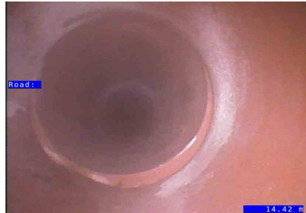
L2X_32a28e5f-1132-4a24-84e6-579a690acda5_20251202_112337_317.jpg, 00:01:52, 14.42 m Joint displaced, medium (between 1.0 and 1.5 times the pipe wall thickness), 3 o'clock to 9 o'clock
