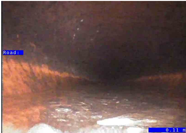
MH1X_058da639-c33a-40be-b1e9-1de6a032ca9d_20251202_105143_363.jpg, 00:00:24, 0.10 m Debris, other, start, Along the bottom of the pipe
