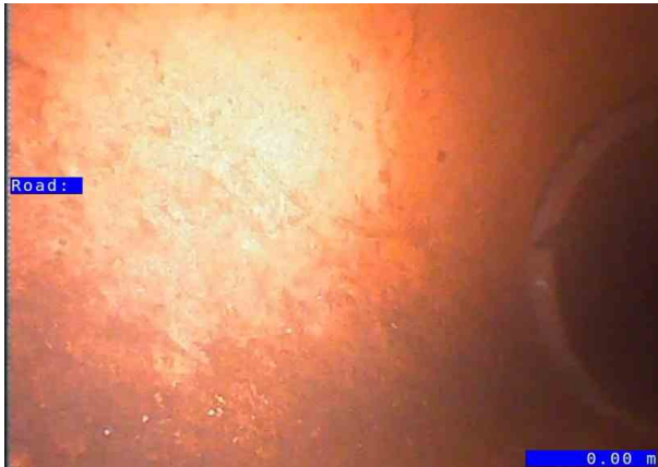
L2X_5591add-9507-4a39-b0dd-ea5071f5684f_20251202_112105_479.jpg, 00:00:09, 0.01 m Joint displaced, medium (between 1.0 and 1.5 times the pipe wall thickness), 12 o'clock to 12 o'clock
