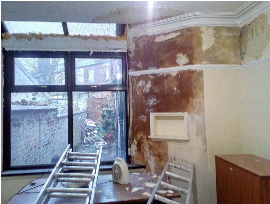
House and garden were in derelict condition with damp issues when we took it over
