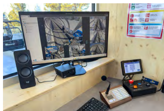
External terminal: Operation and monitoring of the Moving Carpet in the mountain station of an adjacent lift facility
