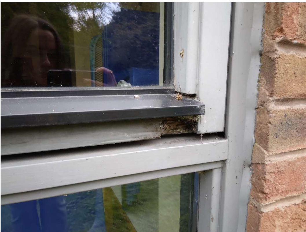
Photograph 8: Damaged timber window
