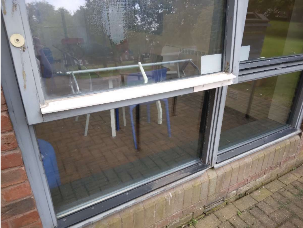
Photograph 7: Previous repair to timber window
