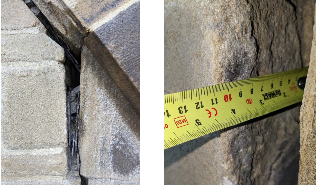
Figure 2-4 Left: Closeup showing slate in joints following raking out of mortar. May imply this has been repointed multiple times. Right: Front stonework 100mm thk only.
