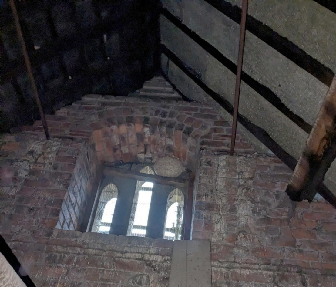
Figure 2-11 Inside attic void (Eastern Gable) showing roof purlins bearing into gable wall & additional tension ties. Inclination not measured nor noticed on original visit.
