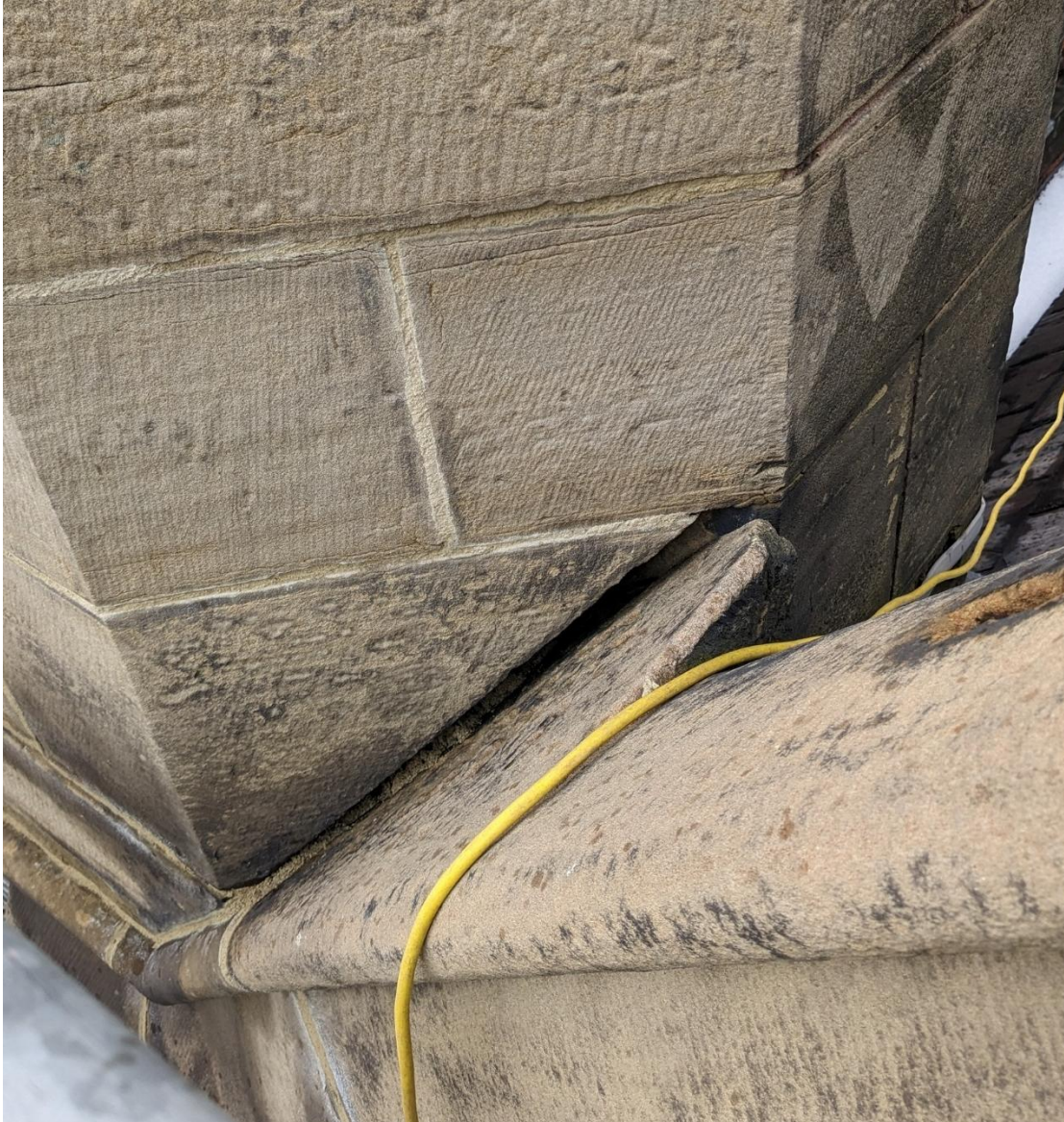
Figure 2-6 2023 photograph- View from the opposite side of the turret showing washed or raked-out mortar. Thought to be fully reinstated in 2024 to prevent water ingress.
