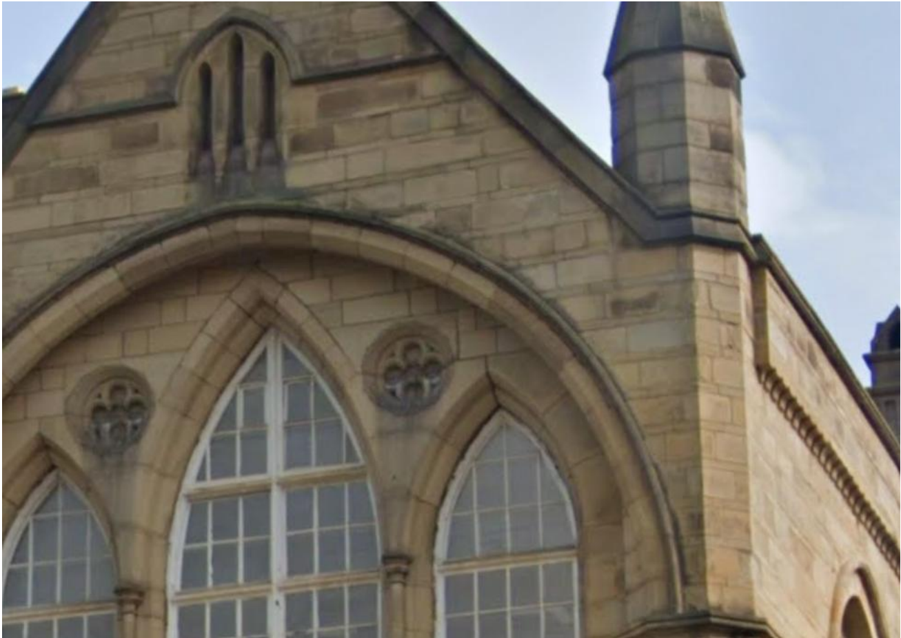
Figure 2-3 Pre Grosvenor restoration works (2021 Google Streetview). This shows mortar in place (too low resolution for observing cracking).
