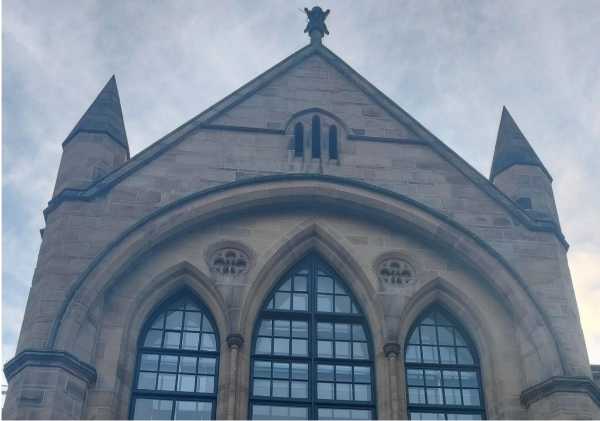
Figure 2-7 Arched Gables to the Grosvenor stone elevation (Eastern Gable- No similar issues evident)
