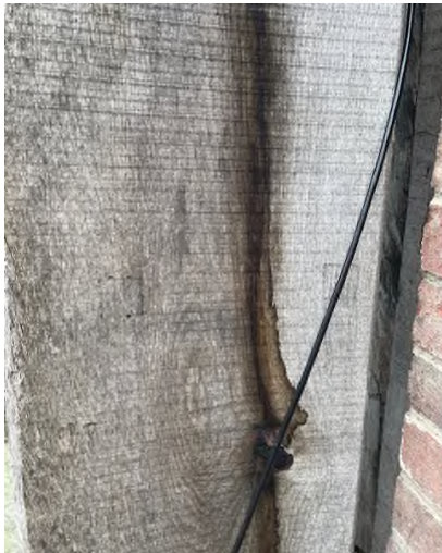
Two small penetrations observed on site from previous timber splice repairs.
