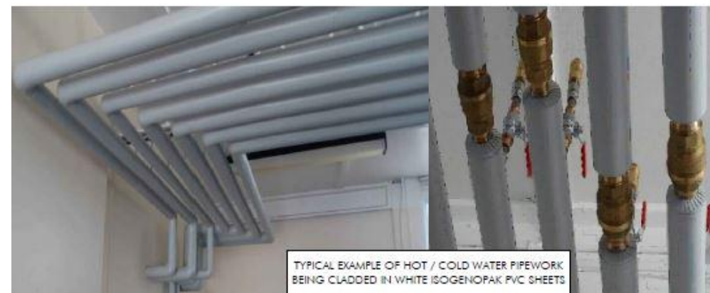
Fig 2: White pipe wrap for exposed water pipework
